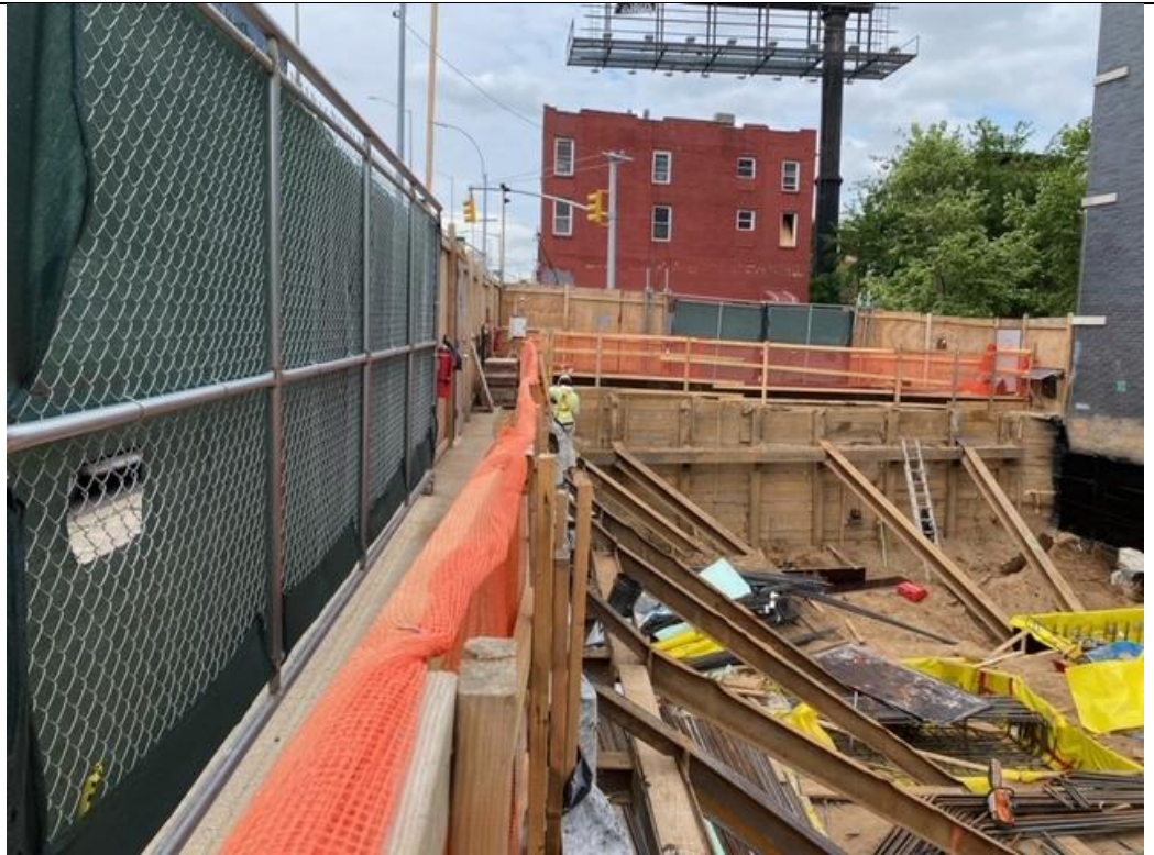
Photo 1 – Facing West CAMP Station 1 in southwest corner, weatherproofin g operations along southern wall.
