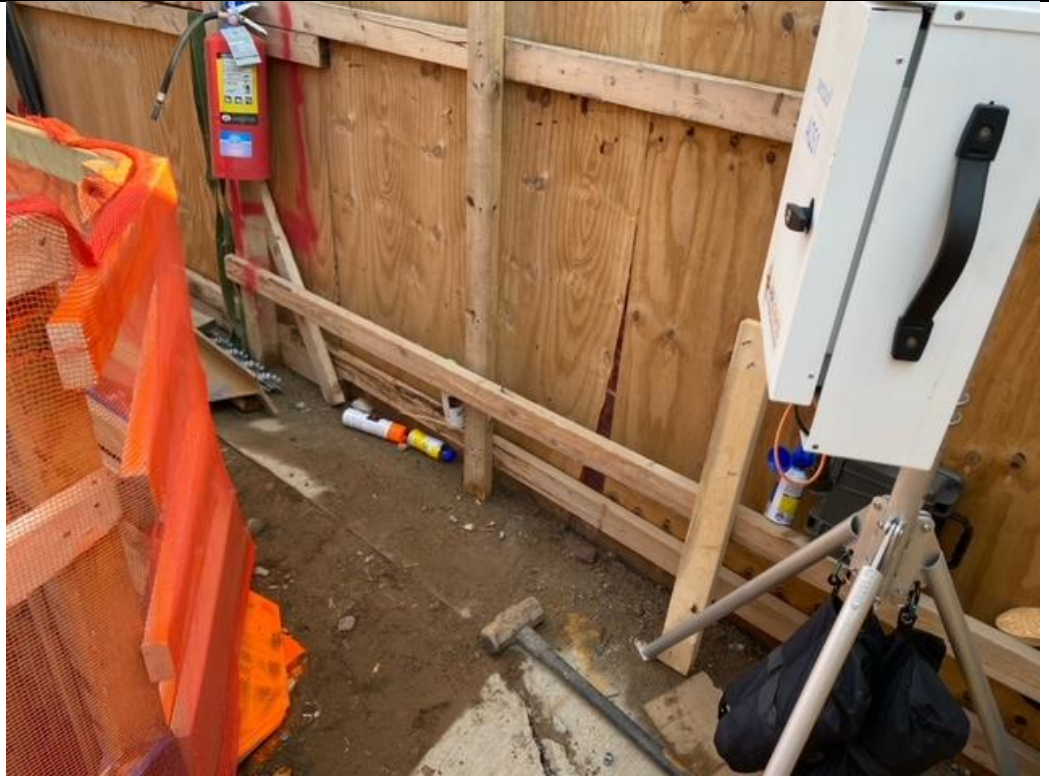
Photo 1 – Facing Northeast VOC exceedance near station 1 due to spray painting.
