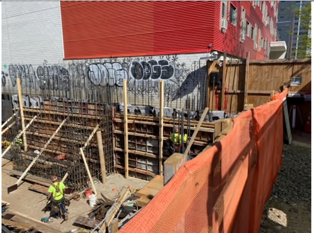
Photo 3 – Facing North Rebar work on north wall, CAMP 2 station located on corner of Site.
