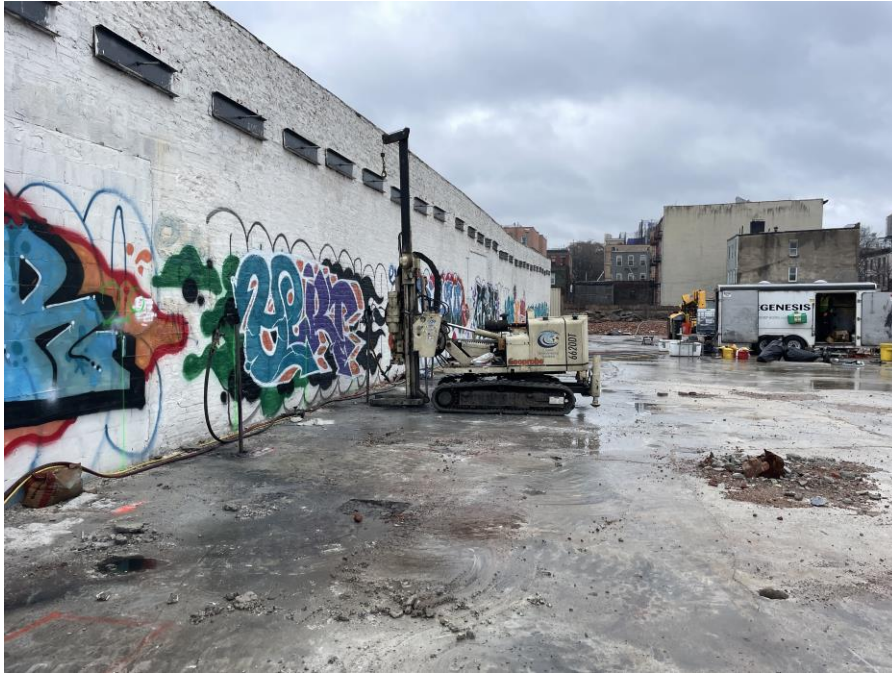
Photo 1: Regensis applying remedial products at injection points IP23 and IP25 (facing east).
