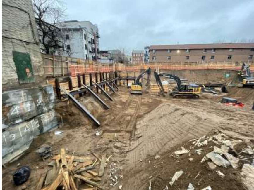
Photo 1: View of Rise excavating and grading native soil for SOE lagging installation in the northwestern part of the site (facing north).
