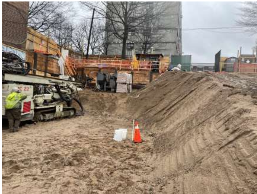
Photo 2: View of a temporary monitoring well MW03 installed by Lakewood (facing south).
