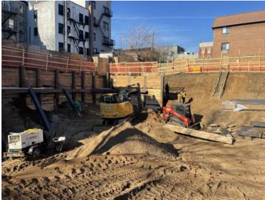
Photo 1: View of Rise excavating native soil for SOE lagging installation in the northwestern part of the site (facing northwest).
