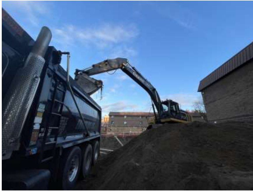
Photo 1: View of Rise loading non-hazardous fill into a permitted tri-axle truck for off-site disposal (facing north).
