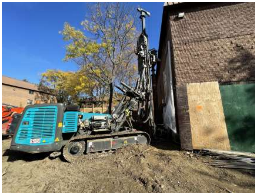
Photo 2: View of Anel installing soldier piles in the eastern part of the site (facing west).
