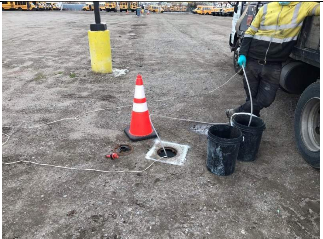
Photo 4 – Developing monitoring well LMW-5 until discharge ran free and clear of solids, facing southwest.
