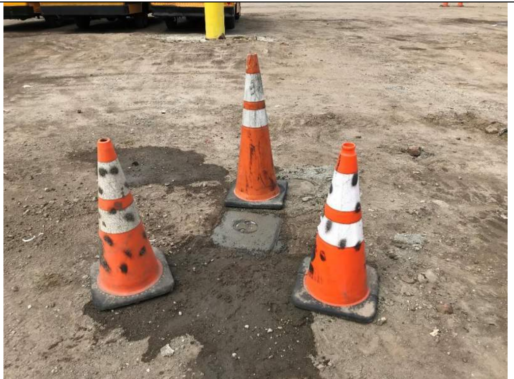
Photo 4 – Completed manhole cover and concrete pad installed at monitoring well LMW-12, facing northeast.
