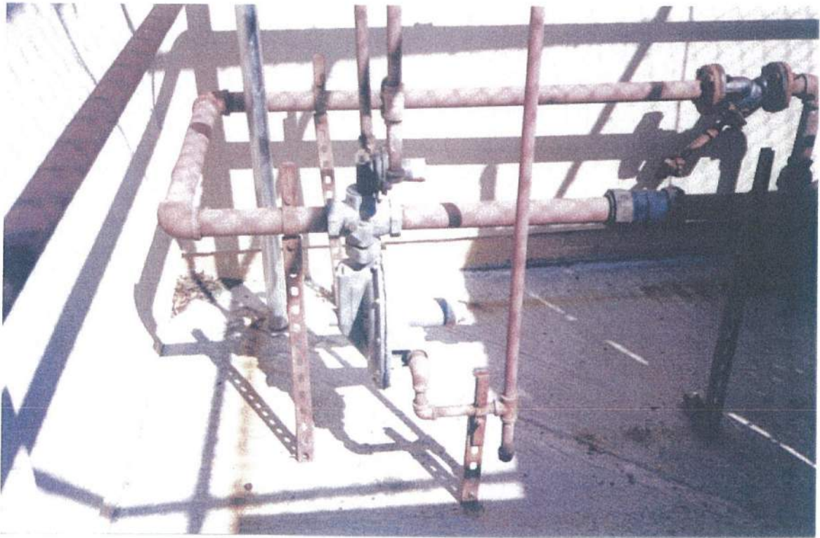
VIEW OF NATURAL GAS METERS
