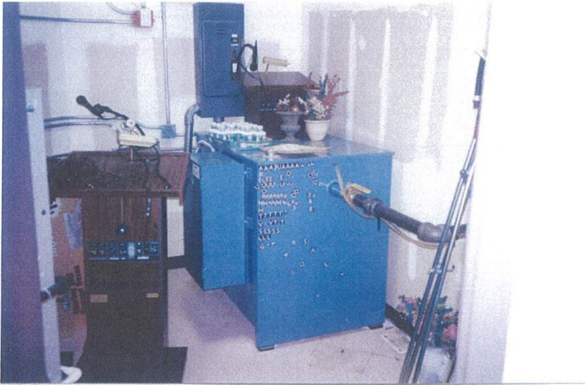
VIEW OF ELEVATOR MOTOR UNIT
