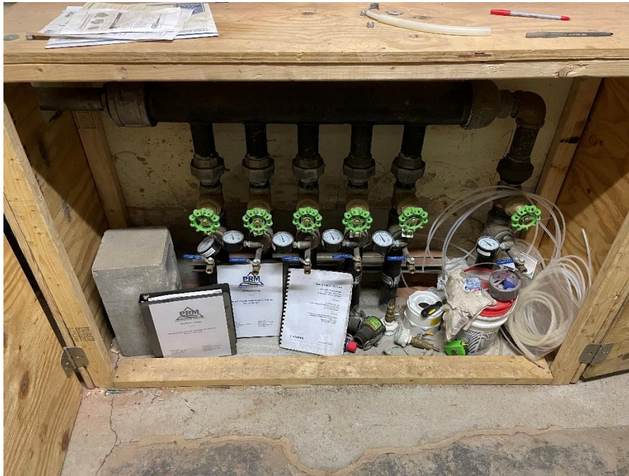
Photo 7, 11/29/2023: View of manifold closet with SVE piping (facing north).
