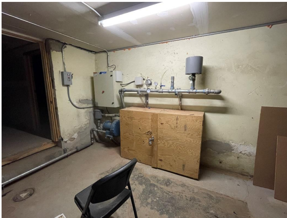
Photo 4, 11/29/2023: View of blower and soil vapor extraction (SVE) system piping (facing northwest).
