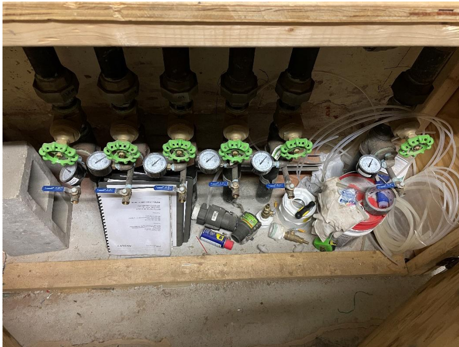
Photo 3, 11/29/2023: View of vacuum gauges (facing down).
