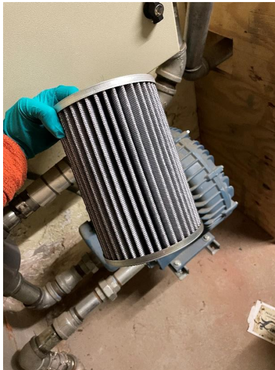
Photo 12, 11/29/2023: SVE blower filter inspection.
