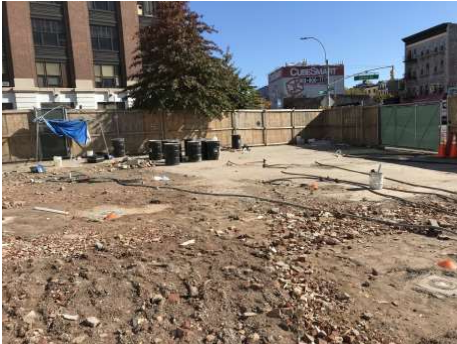
Photo 1: Hoses connected to injection points IP-02, IP-07, IP-08, and IP-12 looking east.
