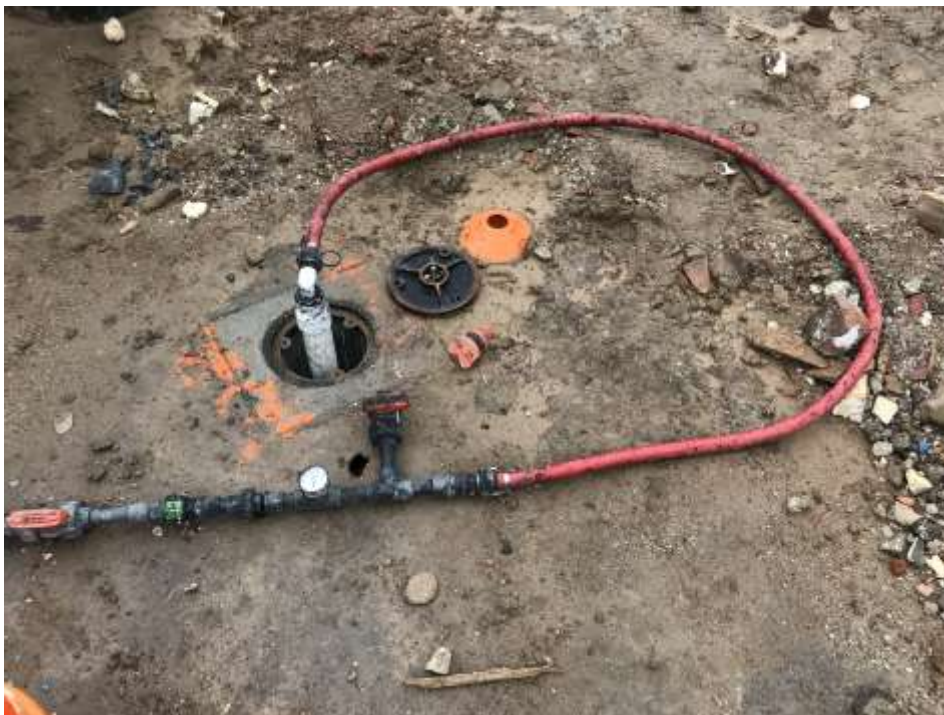
Photo 2: Close up of injection fitting and hose connected to injection point IP-04.
