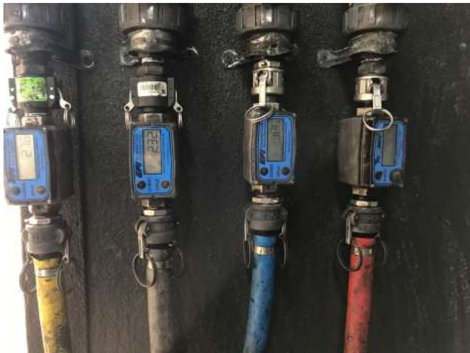
Photo 2: Individual flow meters located inside the trailer, indicating instantaneous and total flow.
