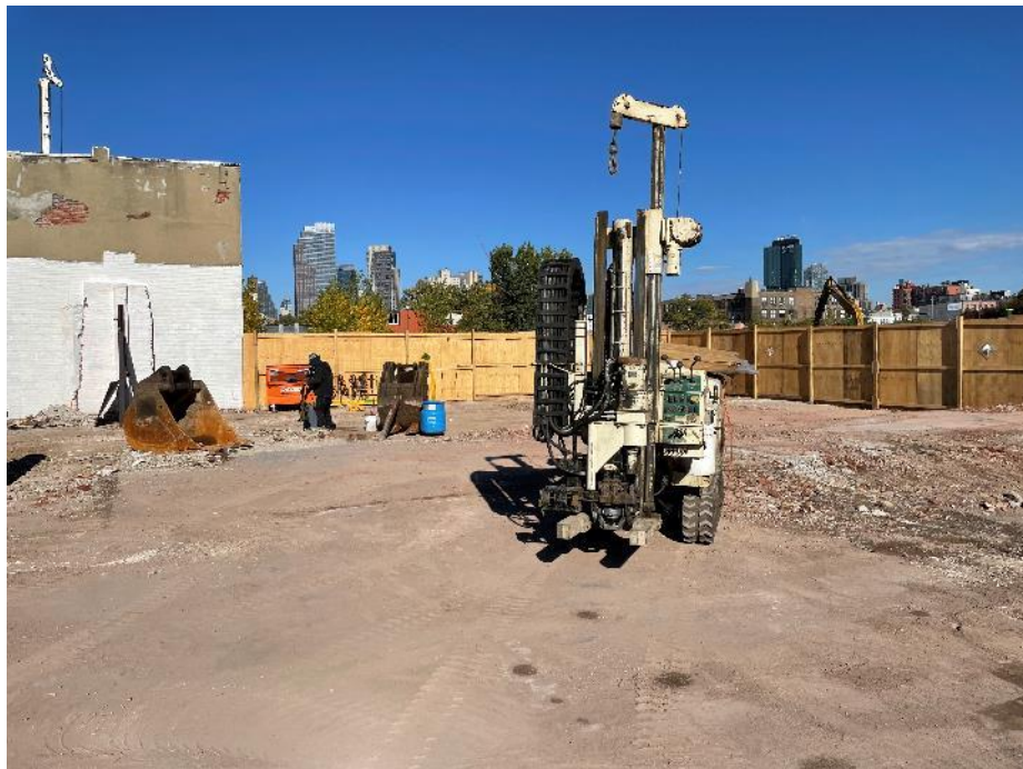
Photo 2: General view of the Geoprobe 6610 DT drill rig in the northern part of the site (facing northeast).
