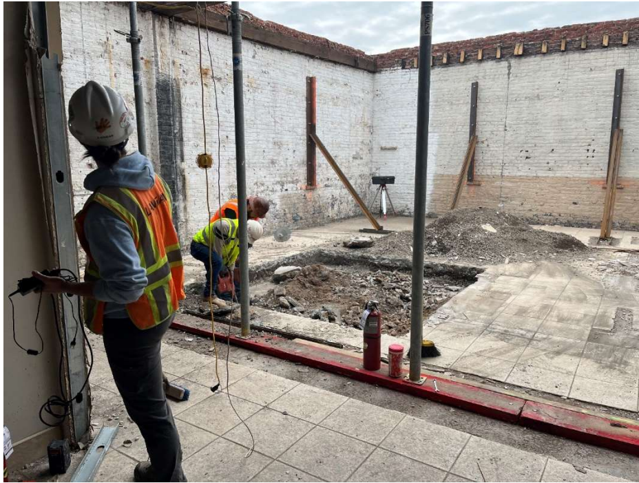
Photo 1: View of the removed concrete slab and subbase (facing northeast).
