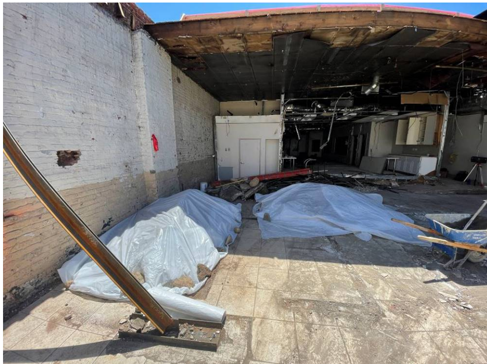
Photo 4: View of soil and gravel subbase stockpiles placed on and covered with polyethylene sheeting (facing west).
