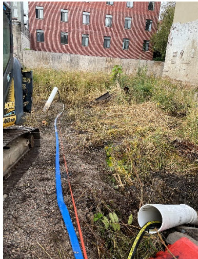
Photo 3: View of the disconnected dewatering suction points.
