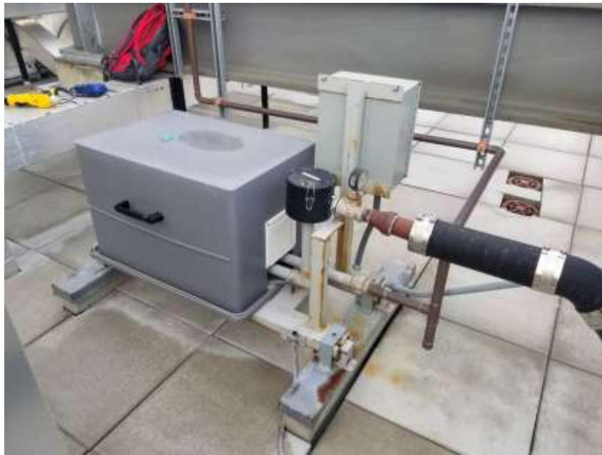
Photograph 7: View of blower box on the roof of the building, facing west (03/31/2022)
