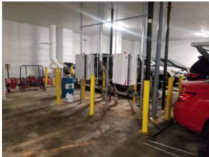
Photograph 4: View of sewer lift system/sump pits and pump located in the cellar level ventilated parking garage (03/31/2022)
