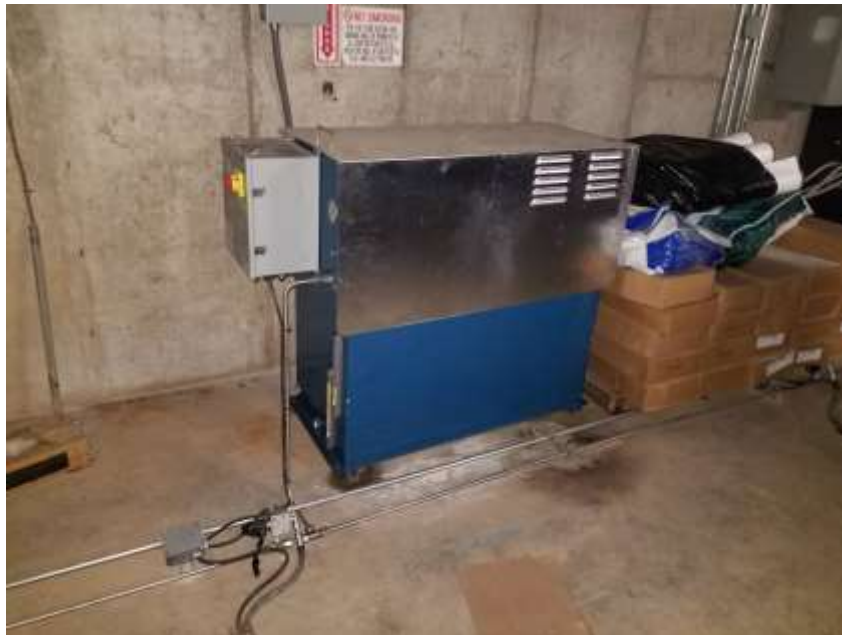
Photograph 5: Area of minor staining beneath the hydraulic oil tank supplying the hydraulic parking stackers observed in the cellar level ventilated parking garage (03/31/2022)
