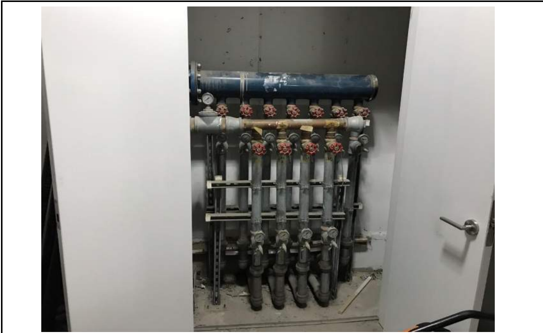
Photo 7: AS/SVE manifold within subgrade parking area, facing west. 6 February 2020.
