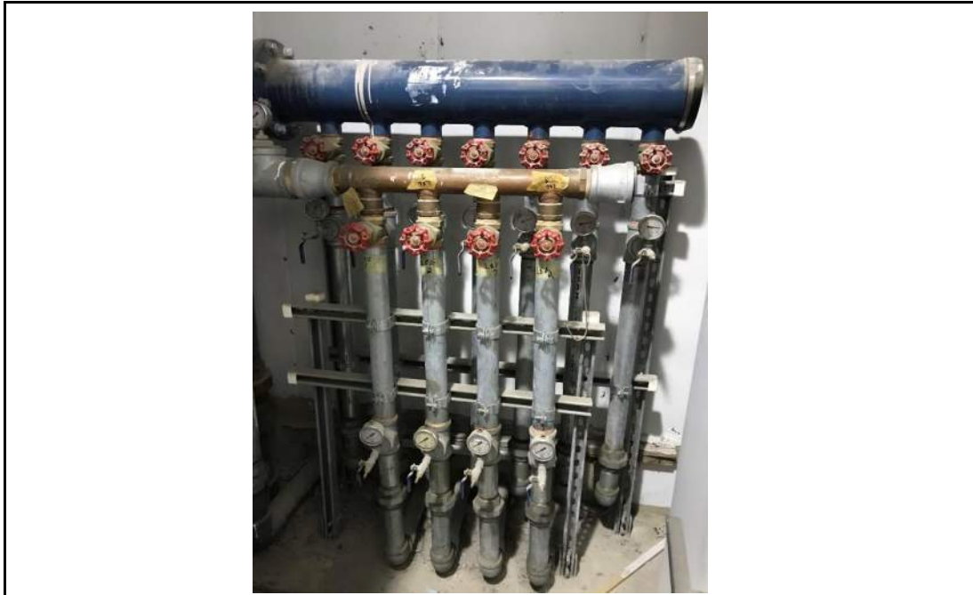
Photo 7: AS/SVE manifold within subgrade parking area, facing west. 21 April 2021.
