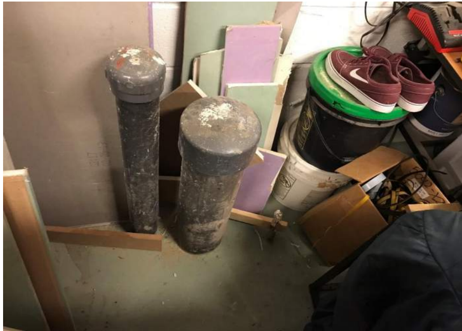
Photo 12: 3-inch air sparge stub and 6-inch multi-phase extraction stub for future connection if groundwater treatment system activation is required, facing south. 6 February 2020.
