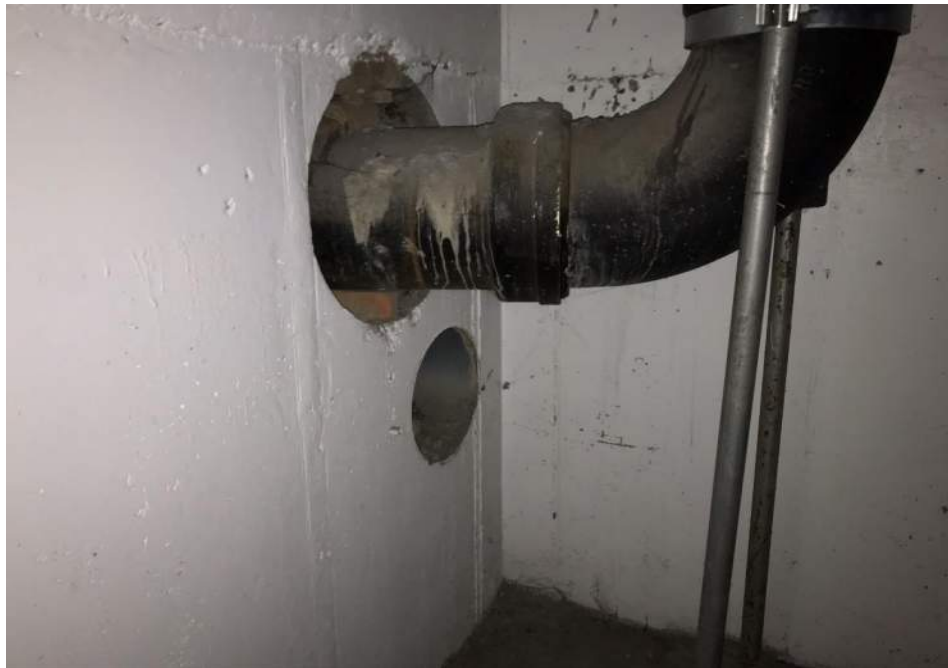
Photo 8: Hole observed in subgrade parking lot concrete foundation wall (beneath the first floor), facing south. 6 February 2020.
