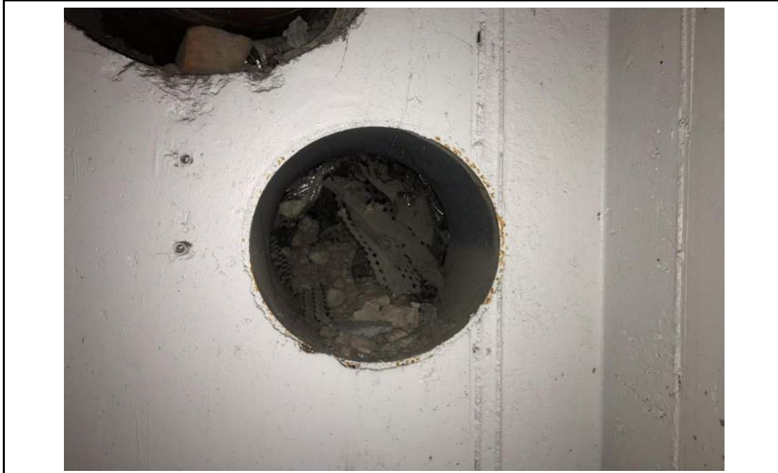
Photo 9: Hole observed in subgrade parking lot concrete foundation wall (beneath the first floor), facing south. 6 February 2020.
