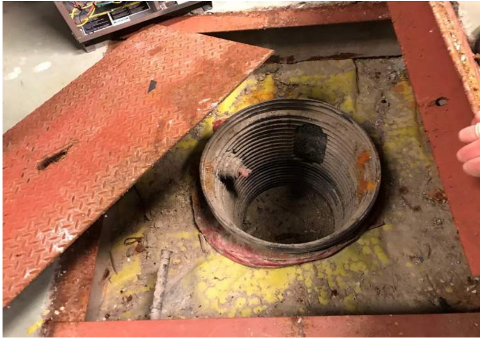
Photo 15: Breach observed in first floor concrete slab surrounding 18-inch sump for groundwater treatment system infrastructure, facing north. 21 April 2021.
