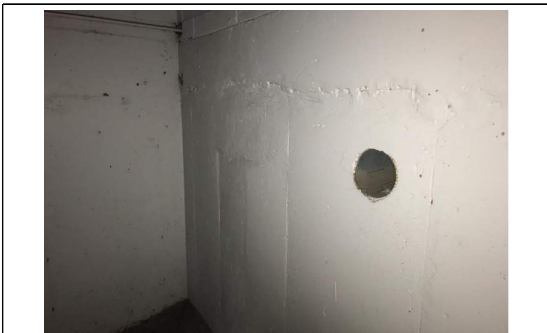
Photo 6: Hole observed in subgrade parking lot concrete foundation wall (beneath the first floor), facing south. 6 February 2020.
