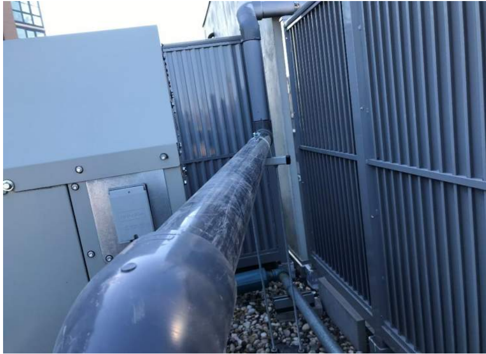
Photo 9: PVC riser pipe rerouting for installation of Obar fan at V3. 30 March 2021.
