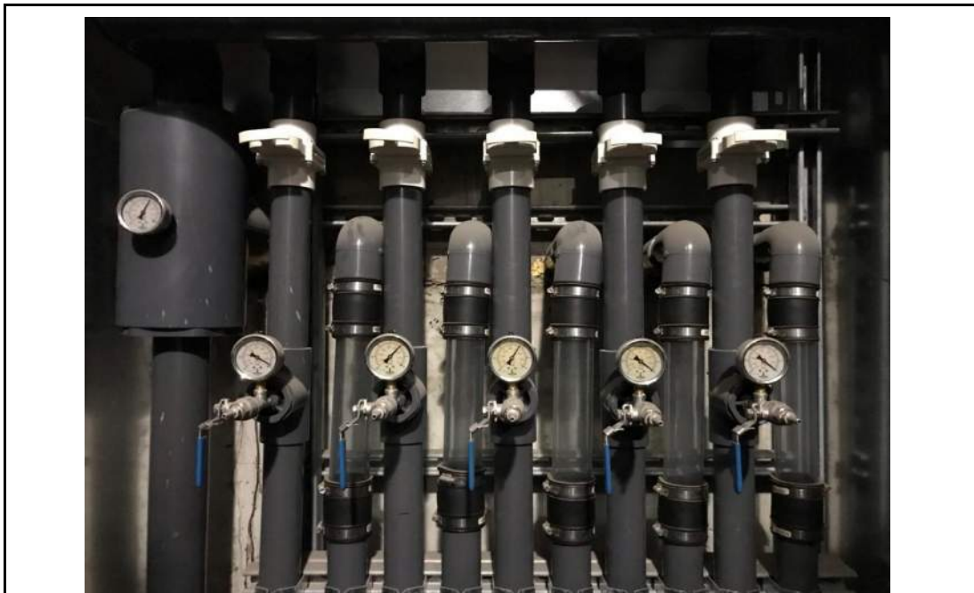
Photo 10: MPE manifold within manifold closet in subgrade parking area, facing south. 21 April 2021.
