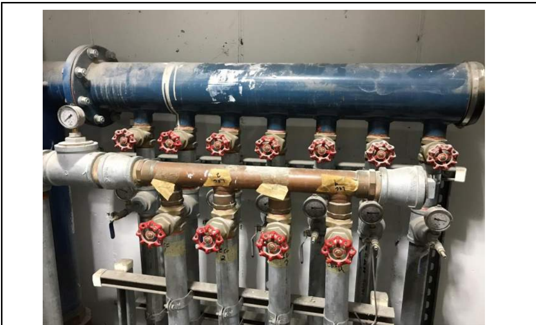
Photo 8: AS/SVE manifold within manifold closet within subgrade parking area, facing west. 6 February 2020.
