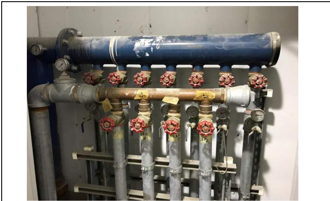
Photo 8: AS/SVE manifold within manifold closet within subgrade parking area, facing west. 21 April 2021.
