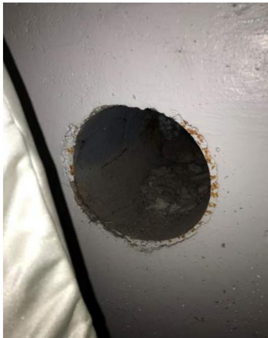
Photo 6: Hole observed in subgrade parking lot concrete foundation wall (beneath the first floor), facing south. 21 April 2021.
