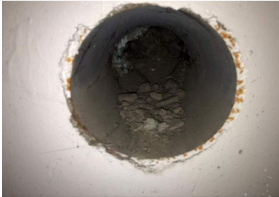
Photo 7: Hole observed in subgrade parking lot concrete foundation wall (beneath the first floor), facing southeast. 6 February 2020.
