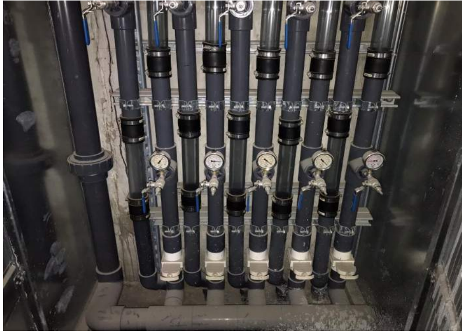
Photo 11: MPE manifold within manifold closet in subgrade parking area, facing south. 6 February 2020.
