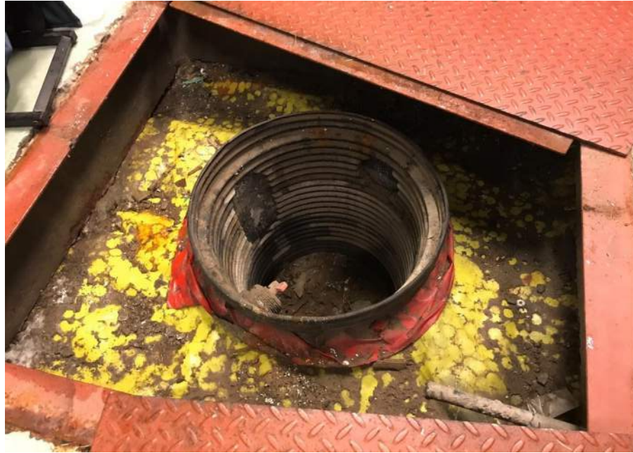
Photo 13: 18-inch sump for future connection if groundwater treatment system activation is required, facing north. 6 February 2020.
