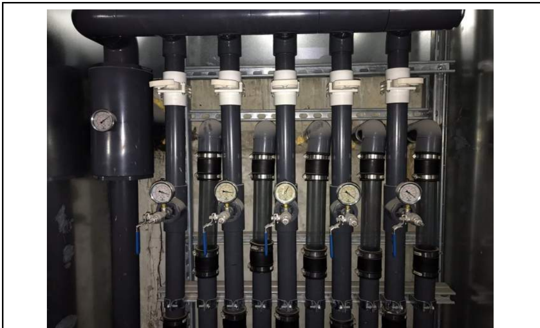
Photo 10: MPE manifold within manifold closet in subgrade parking area, facing south. 6 February 2020.
