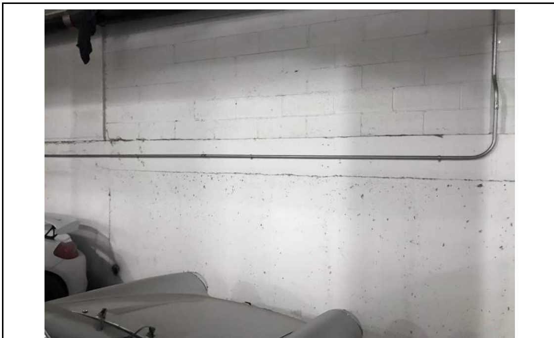
Photo 4: Subgrade parking lot concrete foundation wall (beneath the first floor), facing southwest. 21 April 2021.
