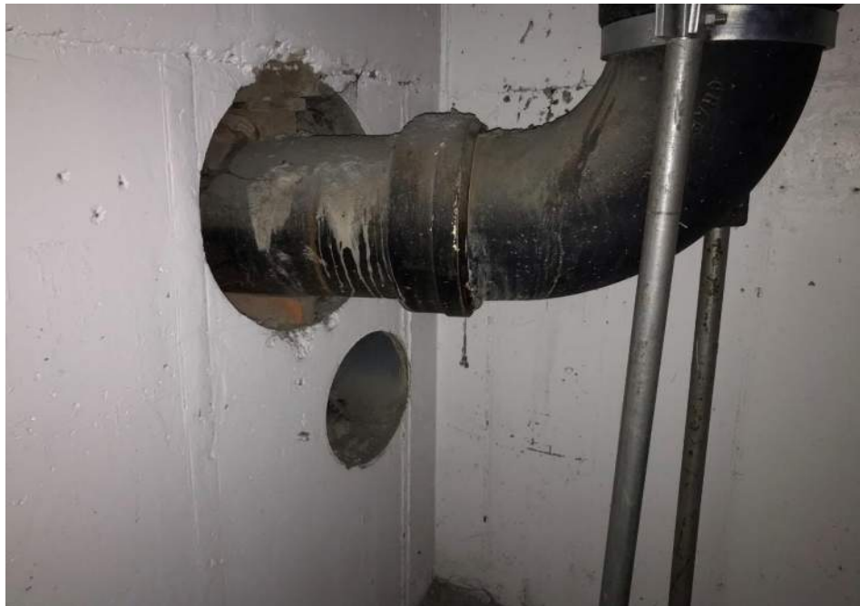
Photo 8: Hole observed in subgrade parking lot concrete foundation wall (beneath the first floor), facing south. 21 April 2021.
