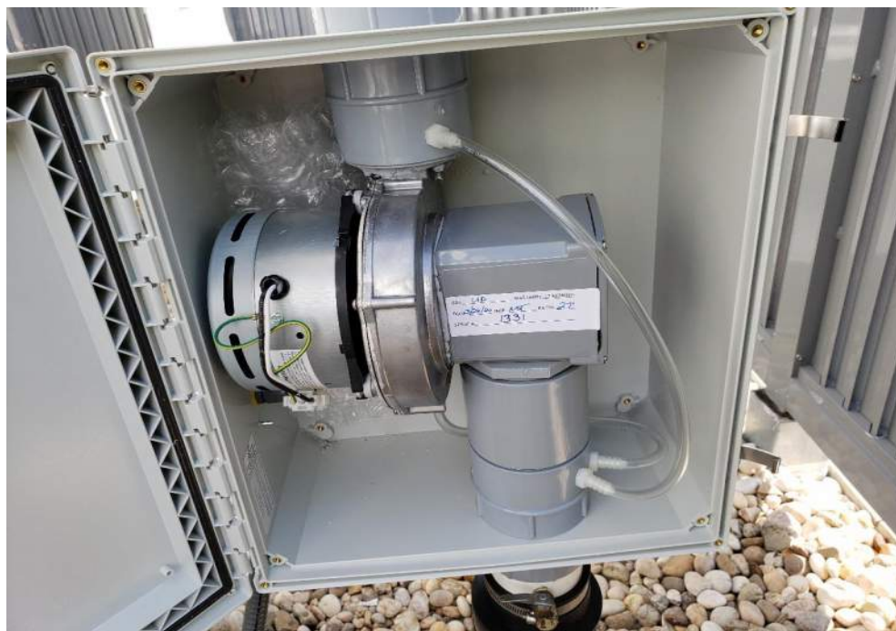
Photo 6: Interior components of V1 Obar fan. 9 October 2020.
