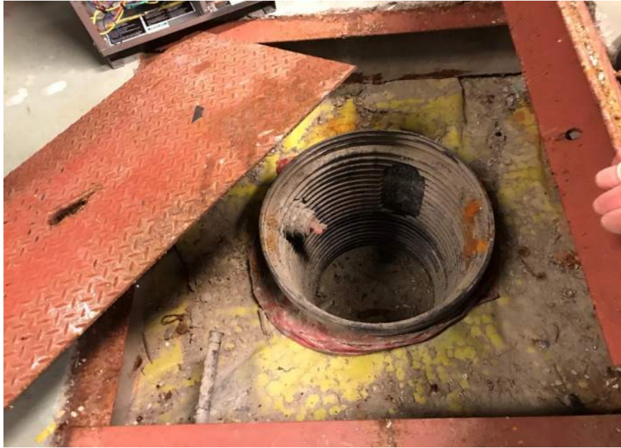
Photo 13: 18-inch sump for future connection if groundwater treatment system activation is required, facing north. 21 April 2021.
