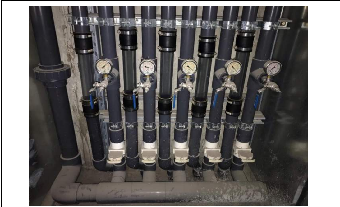
Photo 11: MPE manifold within manifold closet in subgrade parking area, facing south. 21 April 2021.
