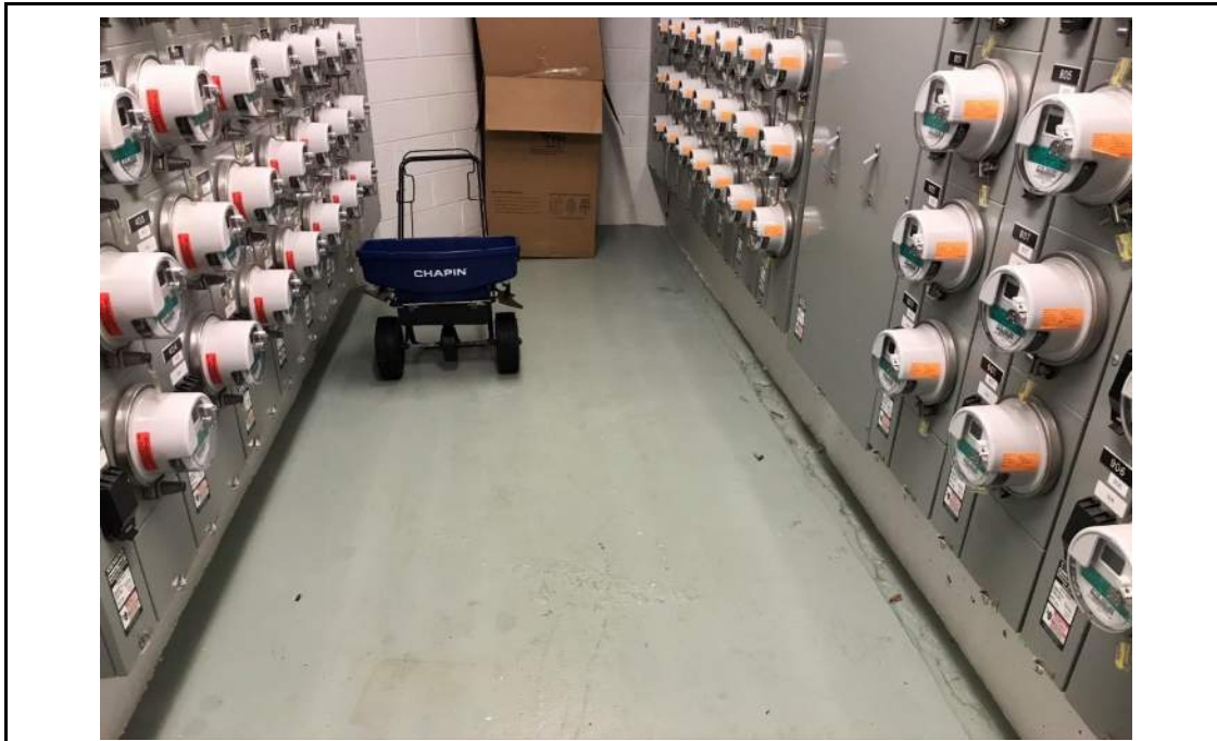
Photo 11: First floor concrete slab in electrical room in the southeastern portion of the building, facing west. 6 February 2020.
