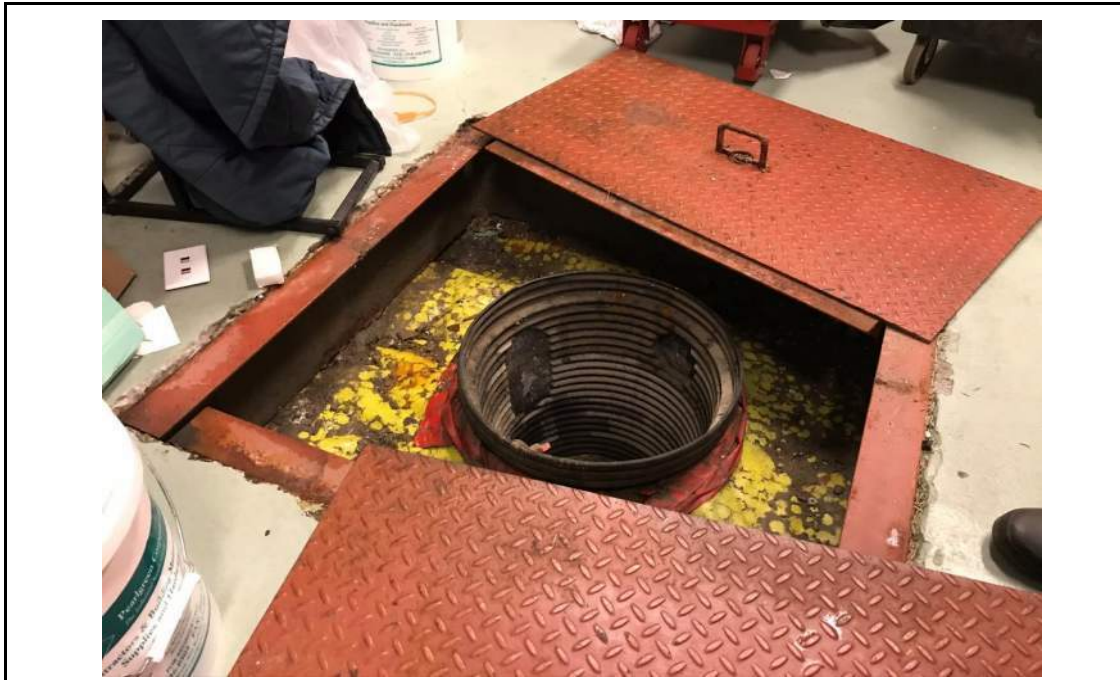
Photo 15: Breach observed in first floor concrete slab surrounding 18-inch sump for groundwater treatment system infrastructure, facing north. 6 February 2020.
