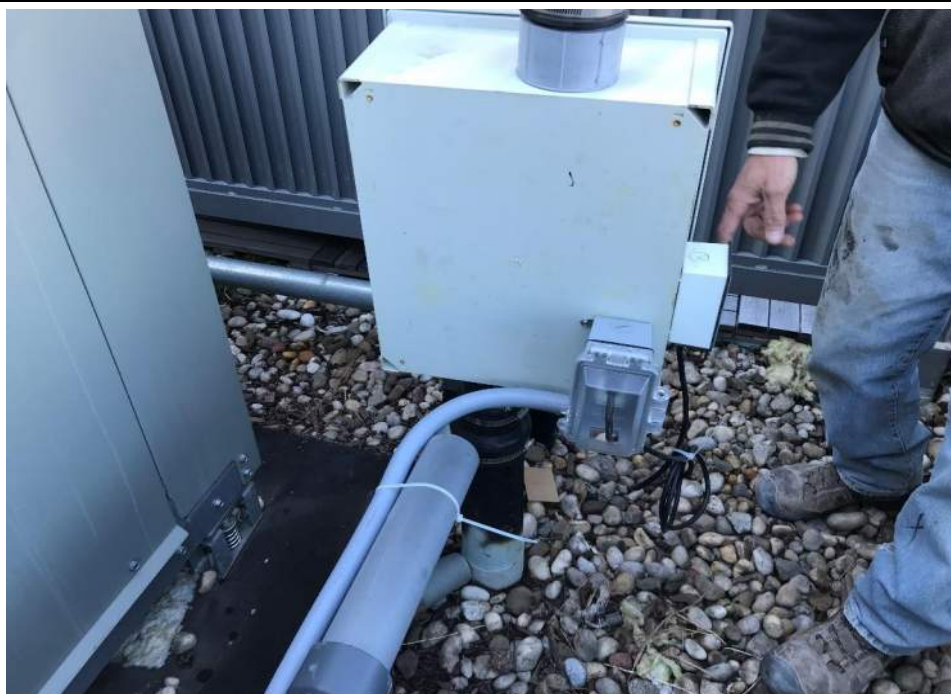
Photo 8: New Obar fan installation at V3. 30 March 2021.
