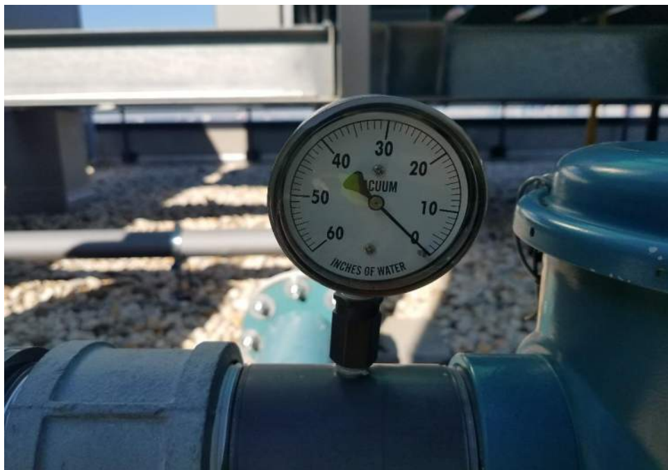
Photo 2: Vacuum gauge at V2. 6 October 2020.
