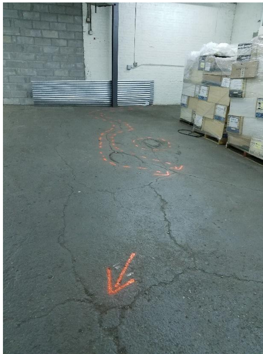
Photo 8: View of the damaged concrete slab in the western portion of Block 4384, Lot 31 (facing west)
