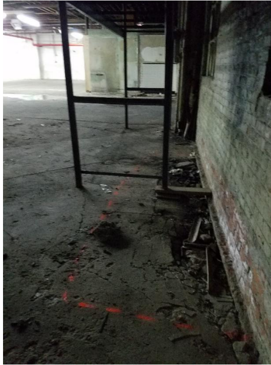
Photo 7: View of the damaged concrete slab in the southwestern portion of Block 4384, Lot 36 (facing east)
