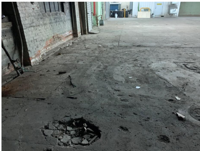
Photo 4: Another view of the damaged concrete slab in the southern portion of Block 4384, Lot 36 (facing north)
