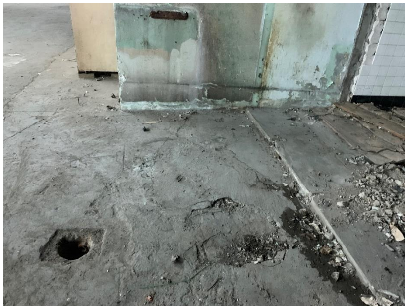
Photo 6: Another view of a former drain with no cover in the southeastern portion of Block 4384, Lot 36 (facing east)
