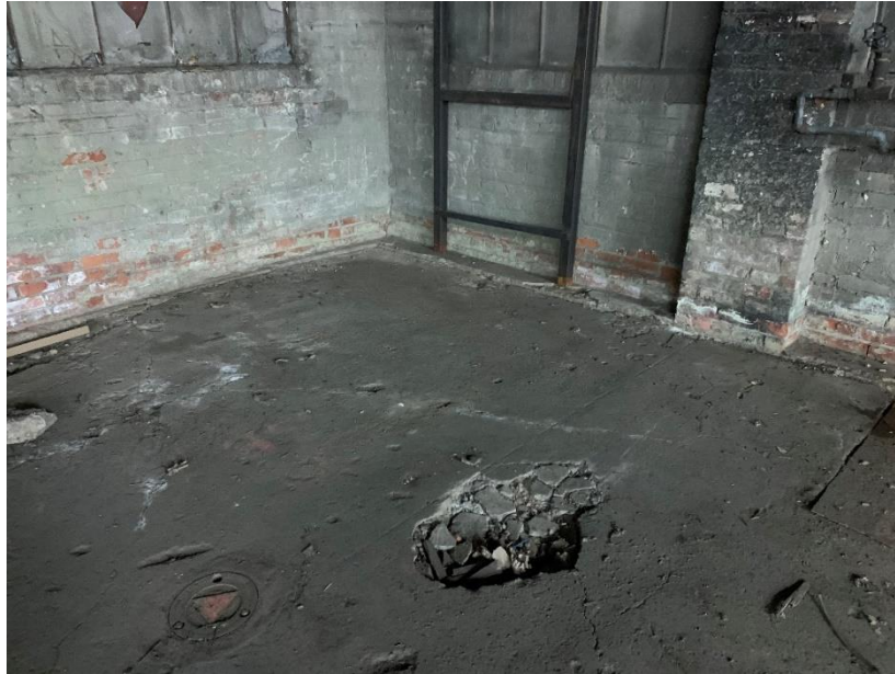
Photo 3: View of damaged concrete slab in the southern portion of Block 4384, Lot 36 (facing south)
