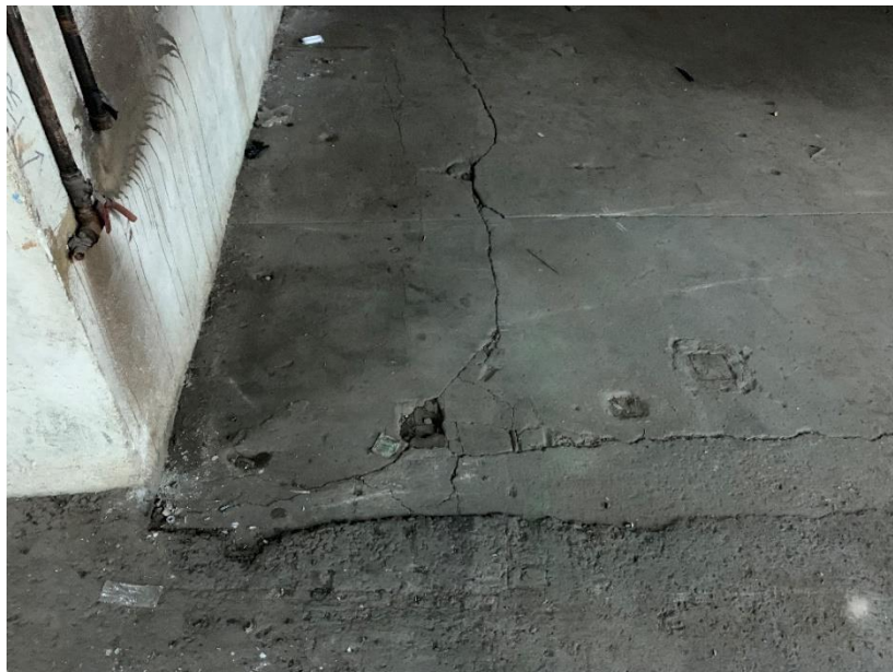
Photo 2: View of damaged concrete building slab in the southern portion of Lot 36 (facing south)
