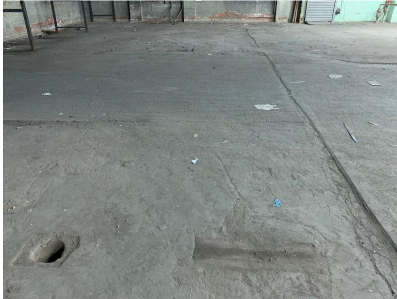
Photo 5: View of a former drain with no cover in the southeastern portion of Block 4384, Lot 36 (facing west)
