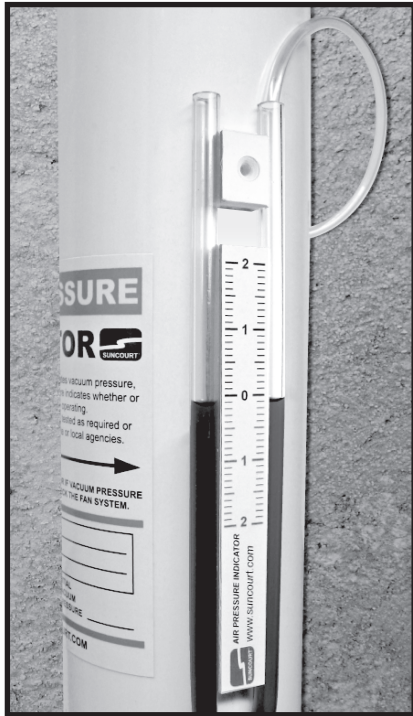
Photo #1 Fan not running
