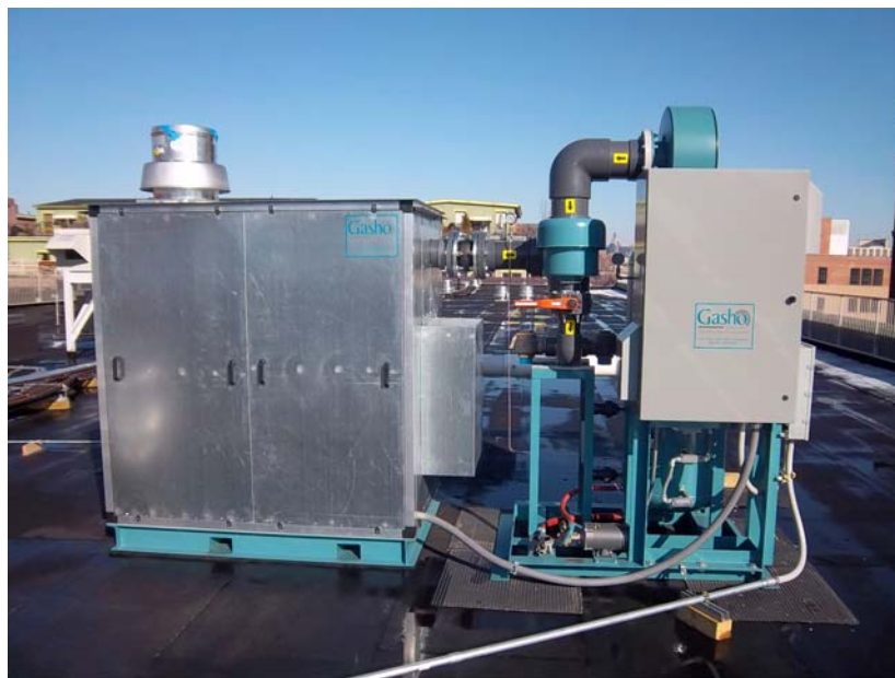
Blower System Mounted on Roof
