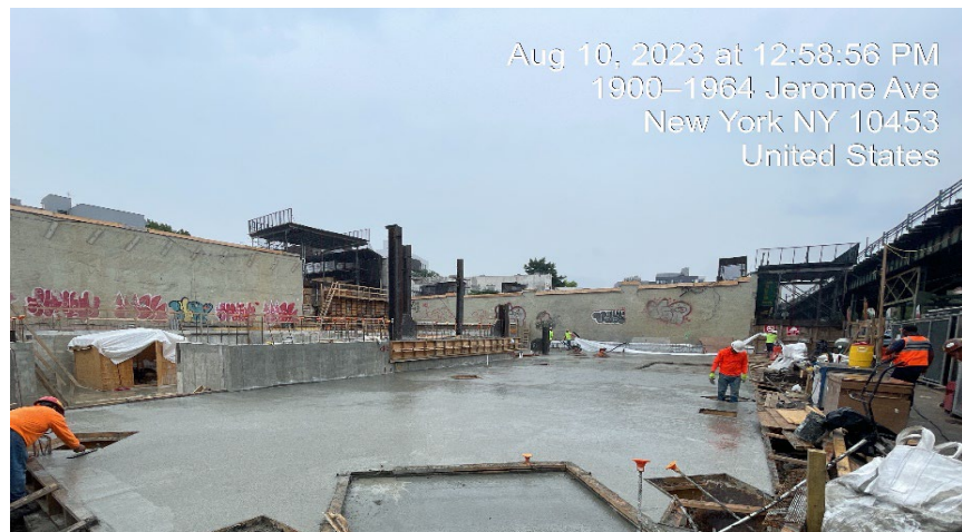
Photograph 3 - A view of the Site with a completed concrete slab. View facing southwest.
