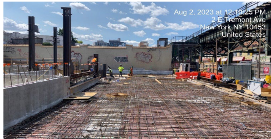
Photograph 3 -View of the metal work being done in WC-03 and the rebar that was previously placed down. View facing west.
