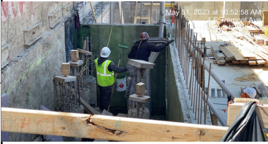
Photograph 2 - Applying glue to the wall to affix waterproofing in WC-04 facing South West
