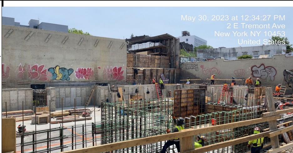
Photograph 2 - Rebar continuing to be installed in grid WC- 03 and WC-04, view facing south east.
