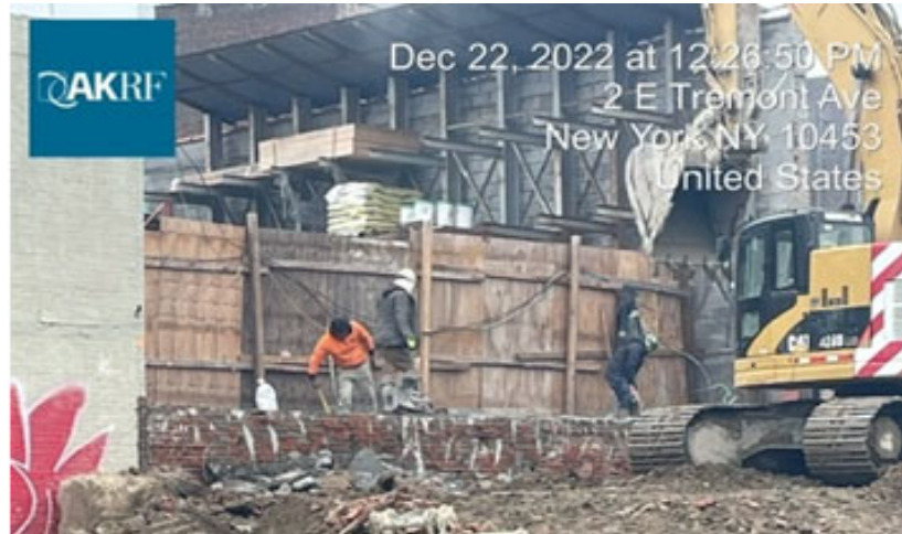
Photograph 2 - The foundation contractor preparing the neighboring site for drilling piles, view facing east.
