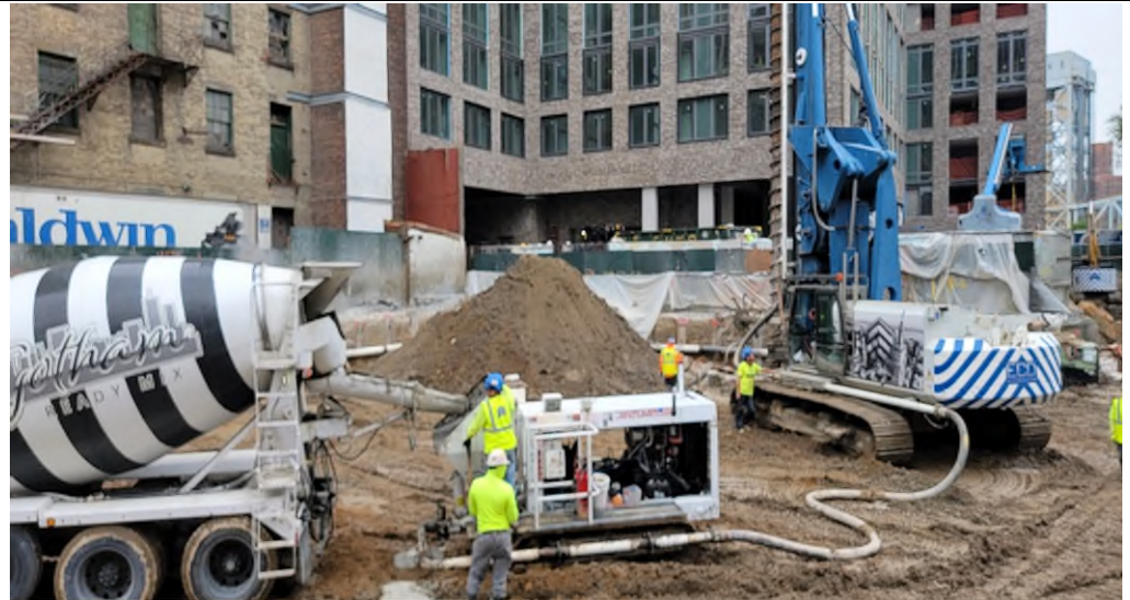
Photograph 2 - ECD drilling piles and pouring concrete in Grid A2, view facing northeast.
