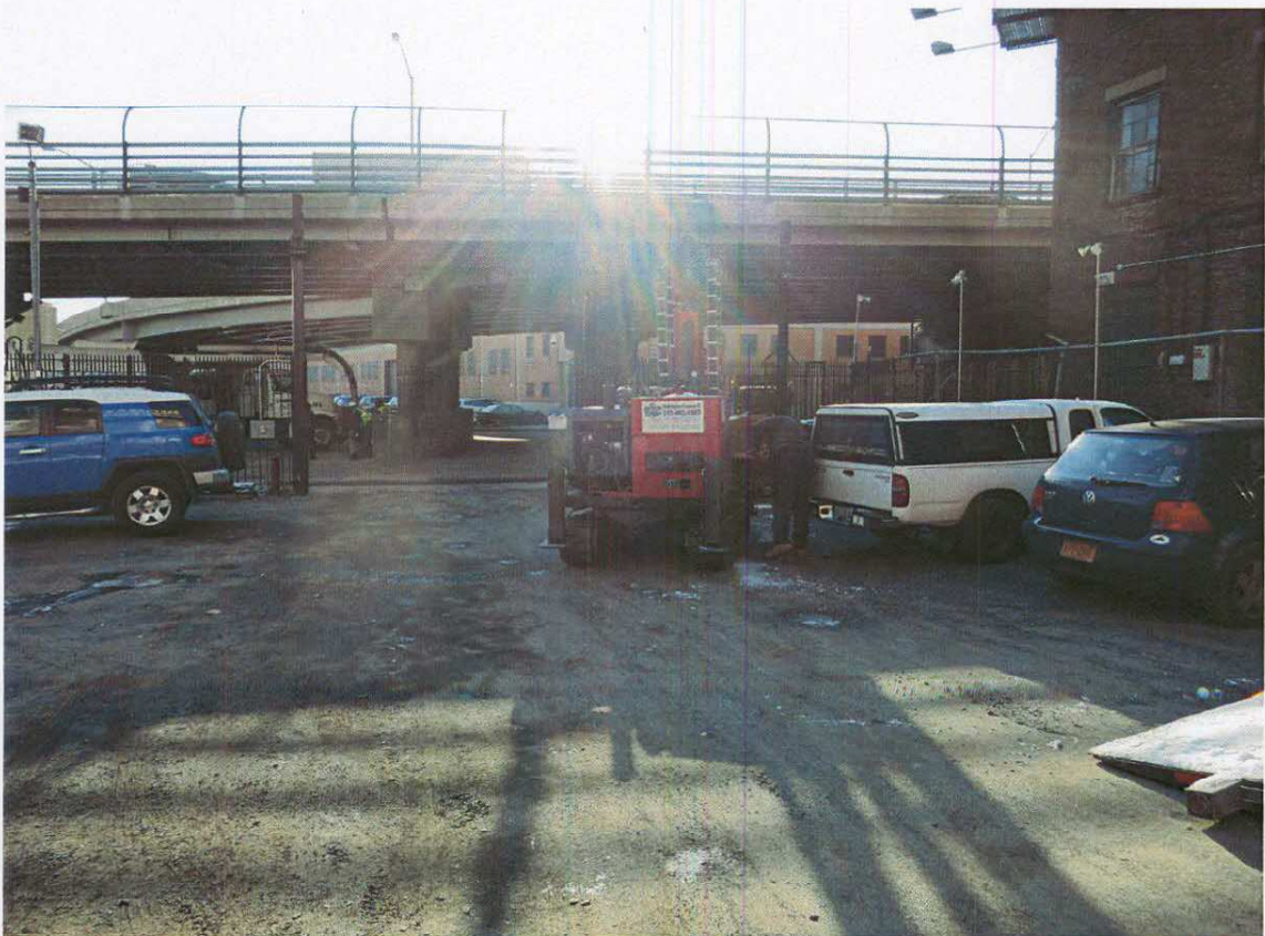
Another View of the Soil Boring Operation at 2413 3 rd Avenue, Bronx, NY
