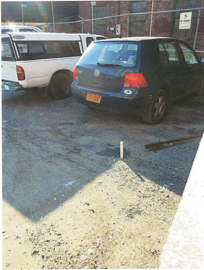
View of the Temporary Groundwater Monitoring Well installed at the Location of Soil Boring #2
