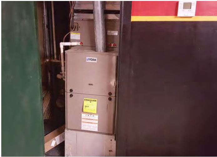
767 E. 133rd St. HEATING UNIT
