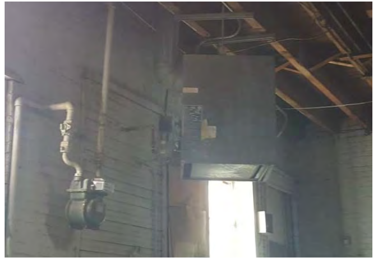
763-765 E. 133rd St. HEATING UNIT
