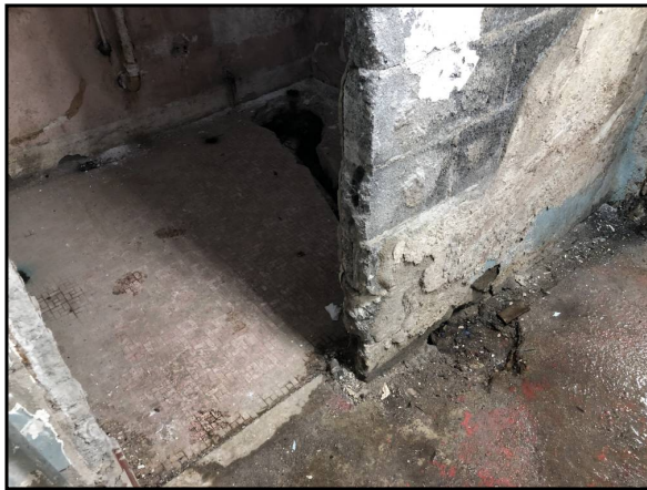
9 : Gouged area of the floor by the bathroom in the basement.
