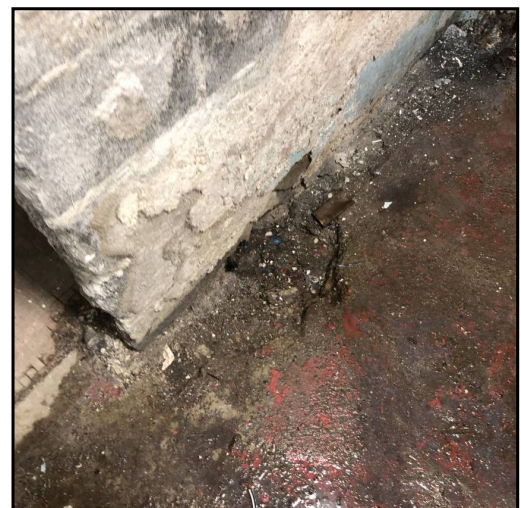
6 : Exposed soils near the bathroom in the basement.
