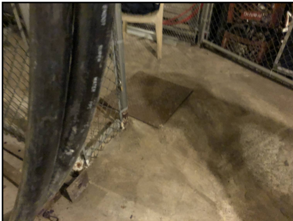
3 : Sump pit with metal cover.
