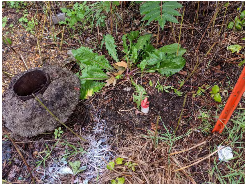
Photograph 5: View of the casing of MW12. Note displaced manhole cover.
