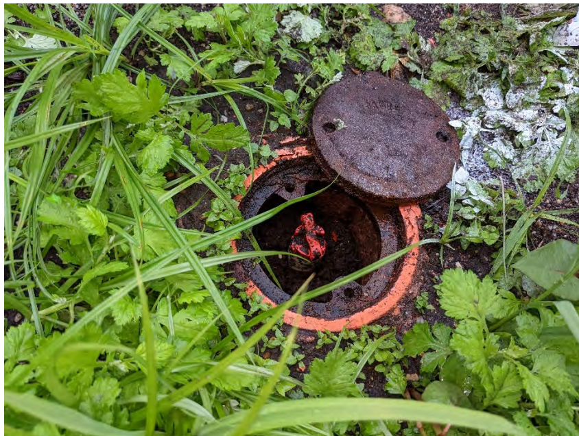
Photograph 10: View of the casing of MW14, which appeared unimpacted by the construction around Smith Pond.
