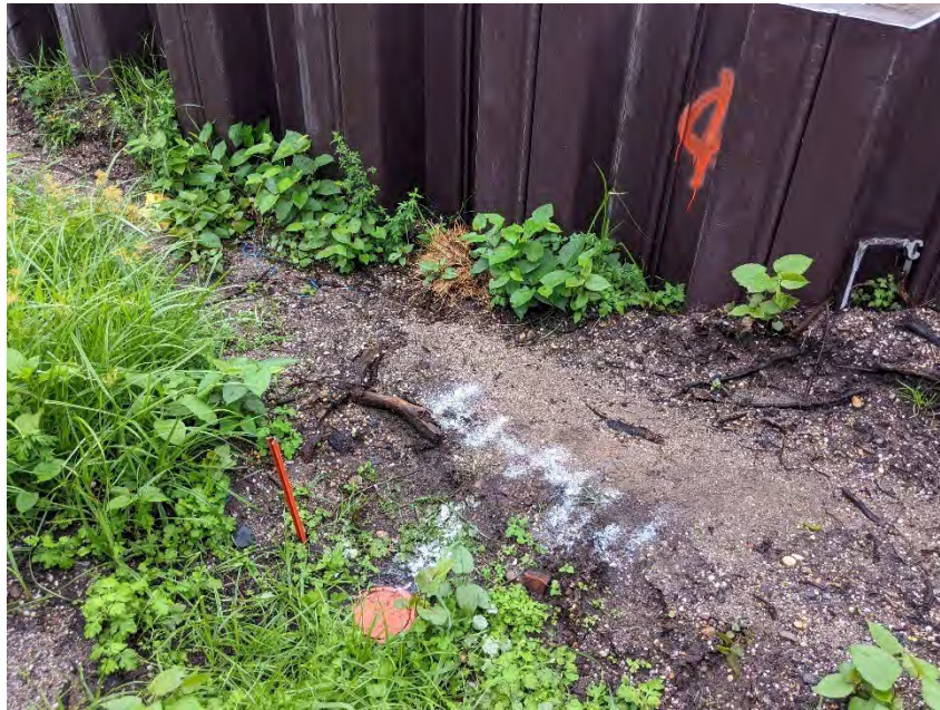
Photograph 9: View of MW14, on the eastern side of the partially installed flood gate.
