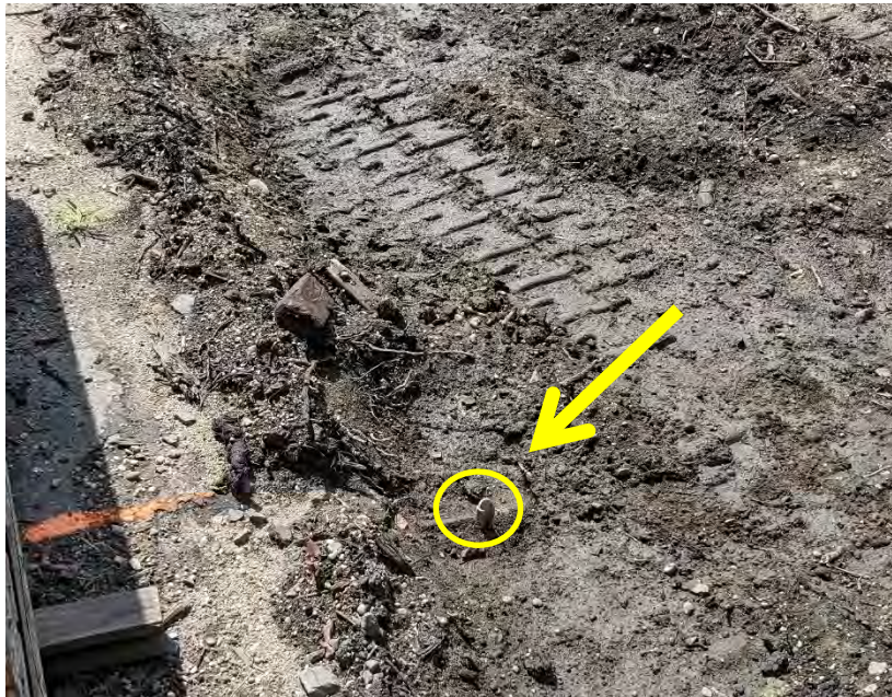
Photograph 13: View of the casing of MW1 during a previous visit on August 31, 2021, which was observed to be broken at the top.
