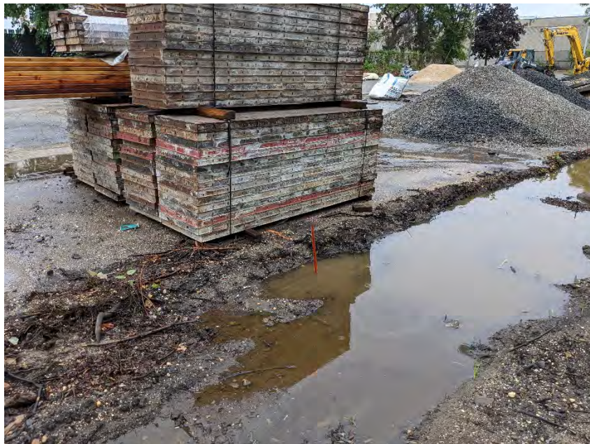
Photograph 12: View of the location of MW1, which was flooded over by the remnants of Hurricane Ida.
