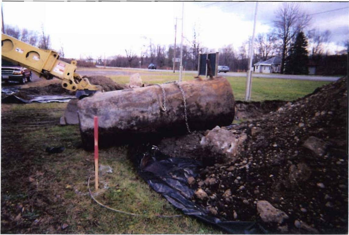
1,000 gallon heating oil UST Note: contaminated soil excavated from the tank pit and stockpiled on plastic.
