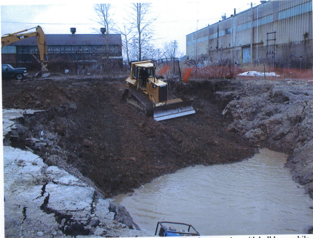
Photo 13: Backfilling excavation with imported clay fill and compacting with bulldozer while dewatering.
