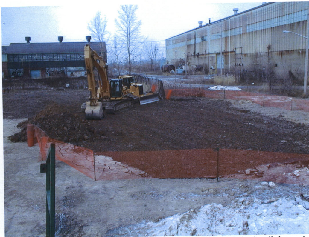
Photo 15: Excavation nearly completely backfilled, temporary fencing being installed around excavation and equipment.
