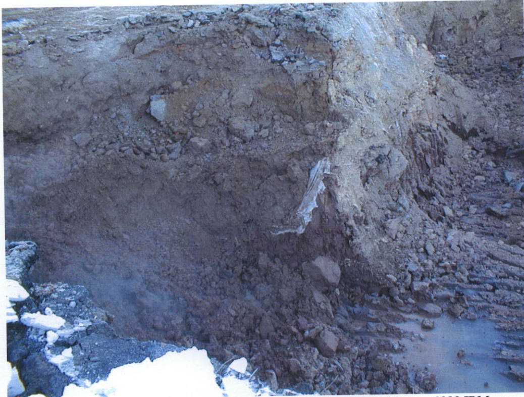
Photo 7: Plastic sheeting can be seen sloping down along the extent of former 1999 IRM excavation.
