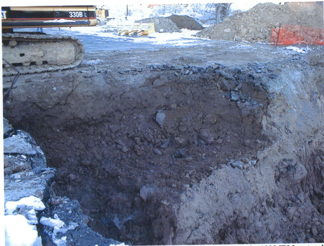
Photo 6: Removing clean backfill from above the plastic sheeting along the 1999 IRM east wall.
