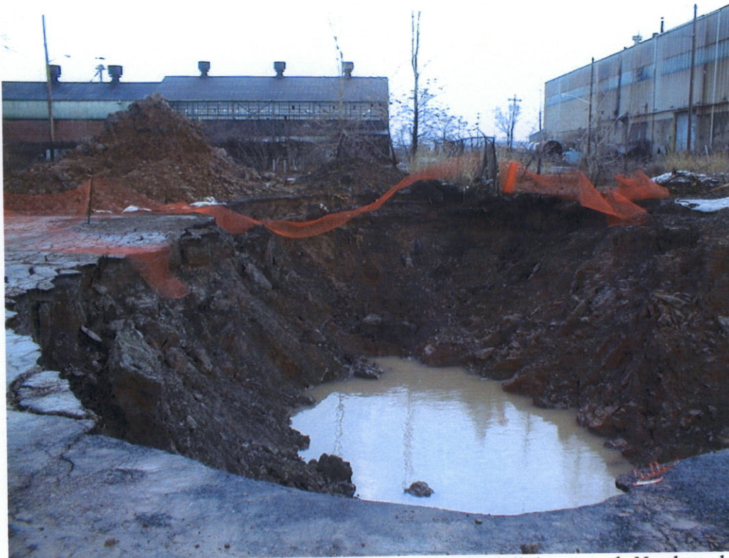
Photo 10: Surface water is accumulating in excavation and sidewalls have caved. Non-hazardous soil stockpiled on plastic sheeting is visible in the background.
