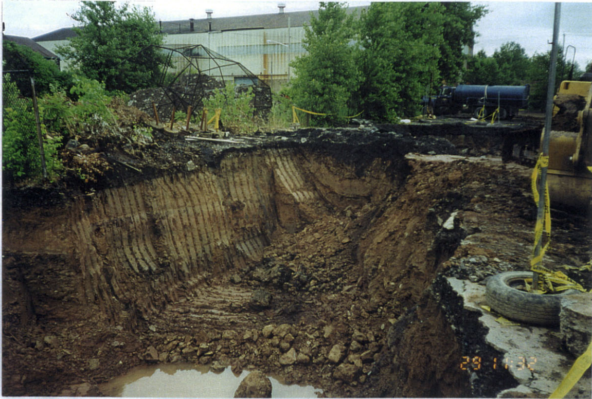
Photo 13: East view of area 1D-extension. This was the former location of the solvent storage cage.
