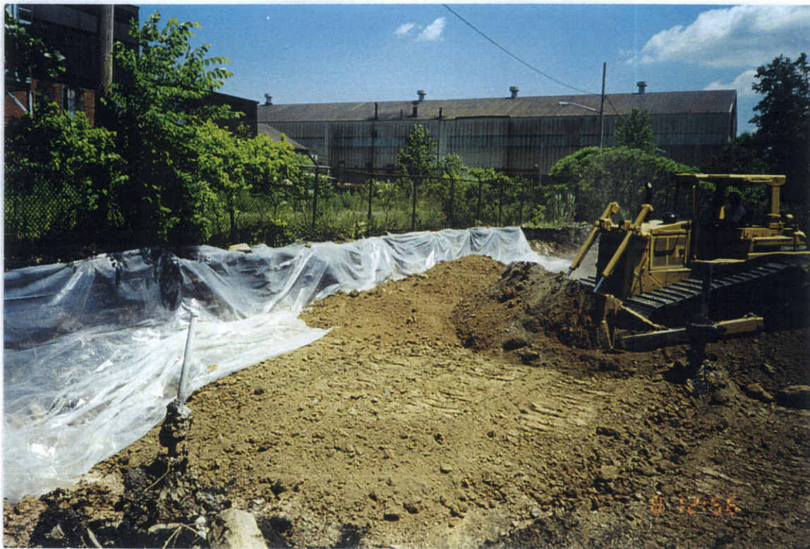
Photo 2: North-east view of backfilling in area 1A. Note plastic sheeting along north wall.
