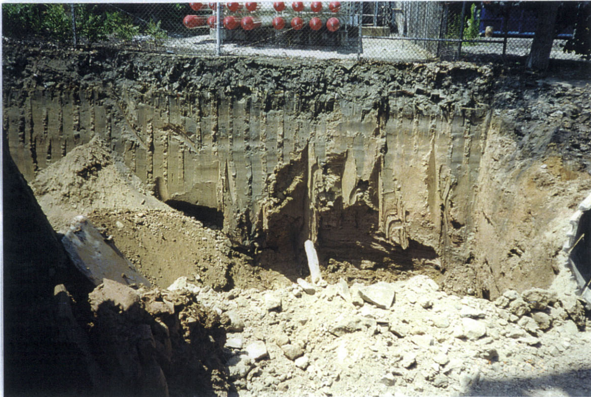
Photo 9: West view of excavation of west wall of area 2A near hydrogen gas cylinders. Excavated as close as possible without compromising safety.
