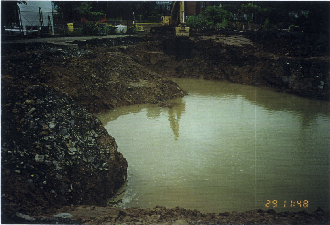
Photo 7: North-west view of west end of area 2A. Note approximately 6 ft of water in excavation.
