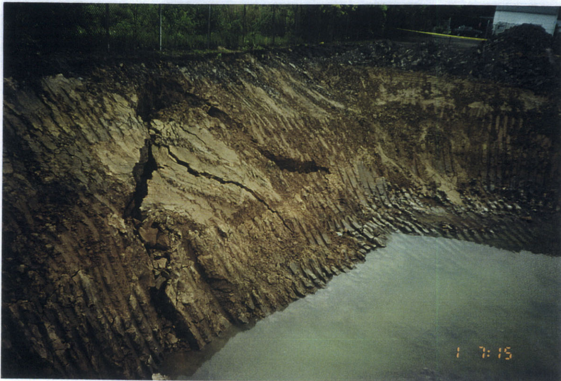
Photo 4: South view along east wall of area 2A where contamination was detected. Note slumping of wall.
