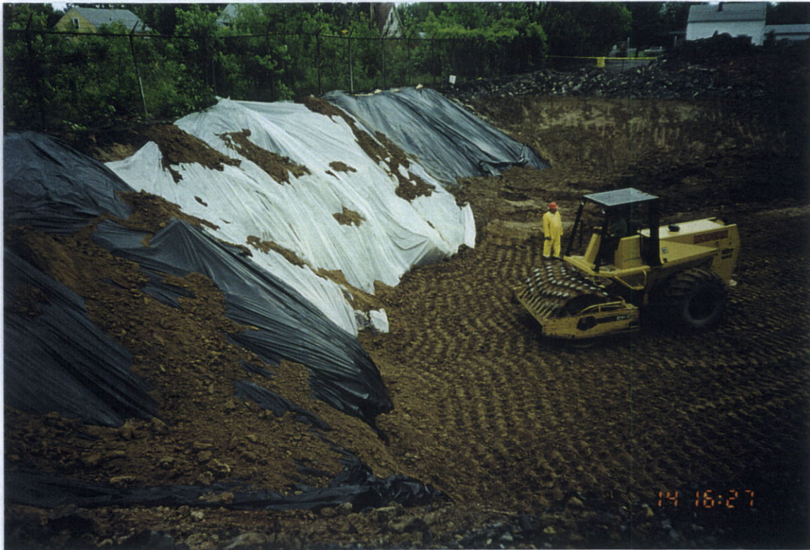
Photo 5: South view of backfilling along east wall of area 2A. Note plastic sheeting along east wall.
