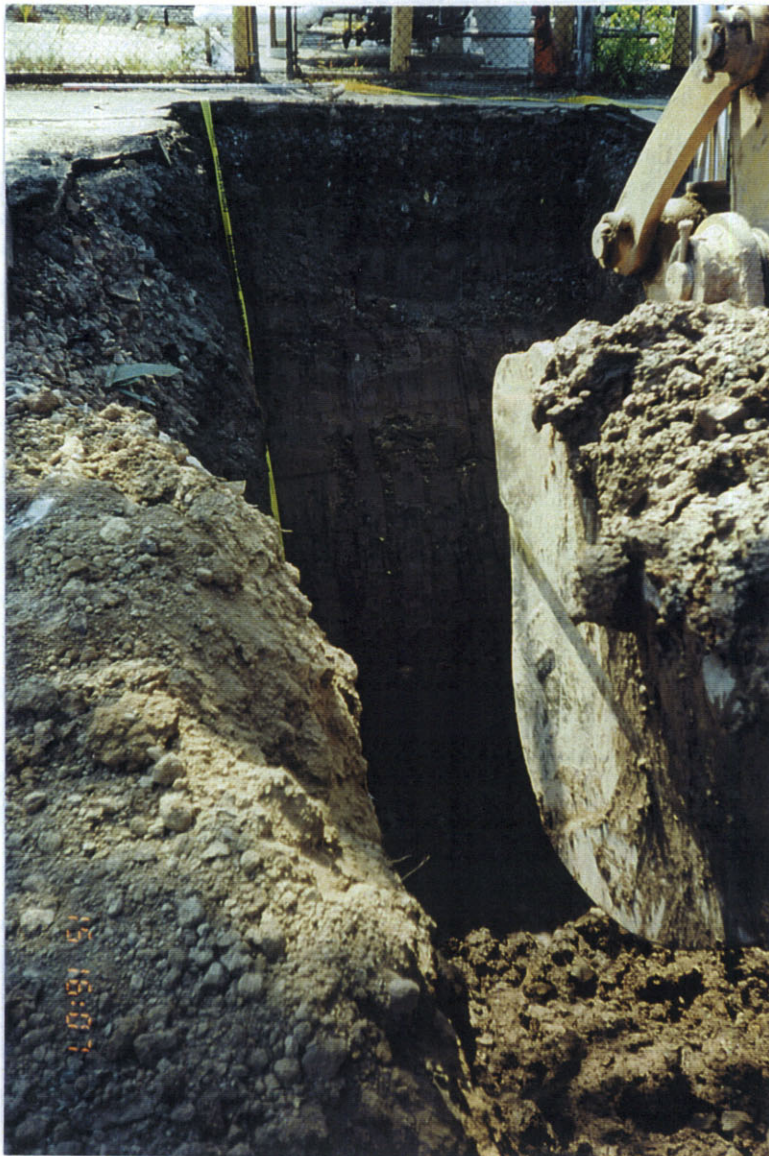
Photo 10: West view of excavation of trench in west wall of area 2A near liquid nitrogen AST. Excavated as close as possible without compromising safety.
