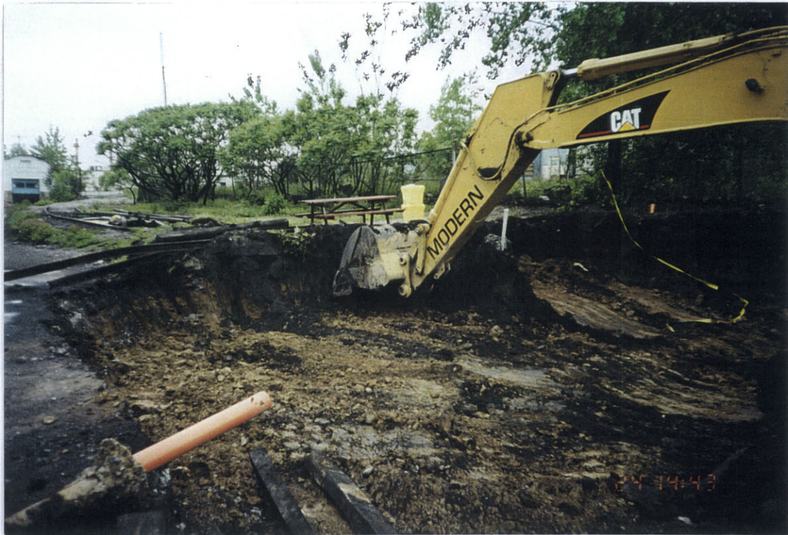
Photo 1: North-west view of area 1A being extended along rail road. Note black PAH staining.
