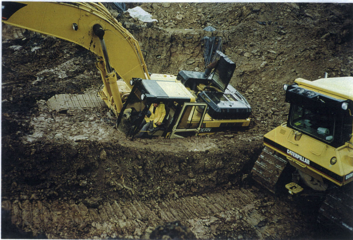
Photo 8: Excavator stuck in soft silt and clay in area 2C.
