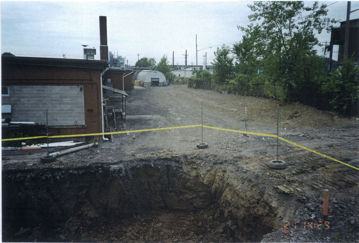
Photo 3: West view of area 1A backfilled and the north half of area 1B excavated.
