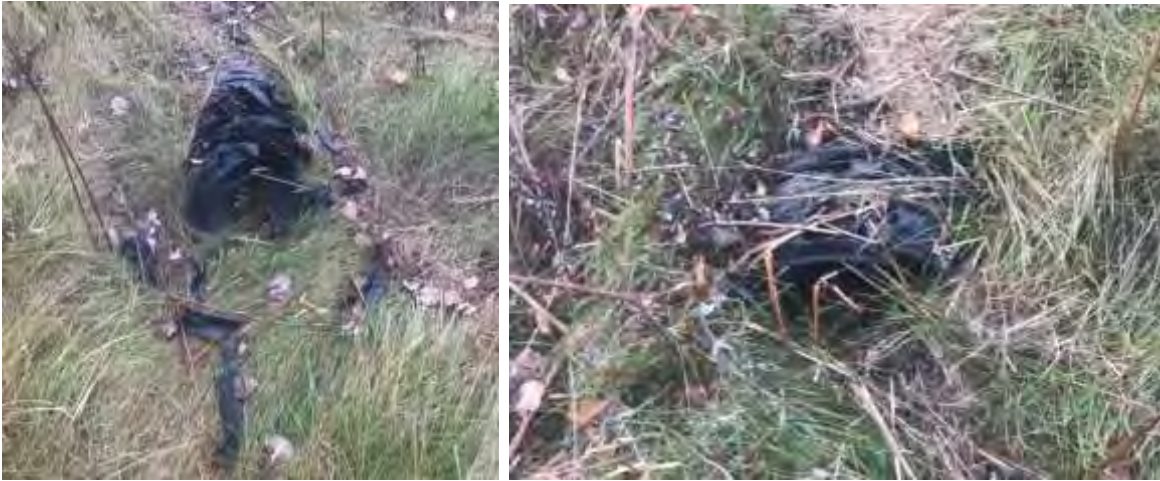
Stormwater drainage plastic culvert, minor damage, no standing water 10/26/20 NWP
