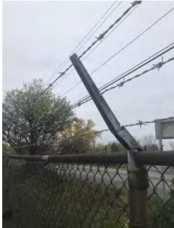
New barbed-wire along northern portion of Witmer Rd. fence, good condition 10/26/20 NWP
