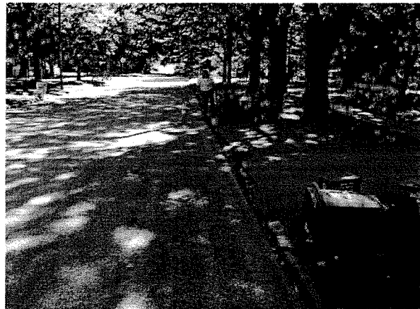
The traffic cone on the right marks the Monitoring Well (MW) that was damaged by the milling machine
