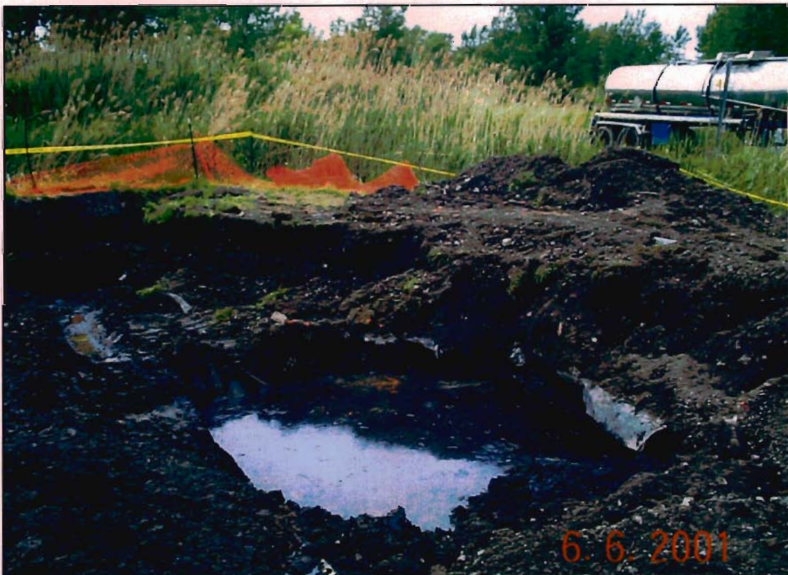
Groundwater seepage into excavation.
