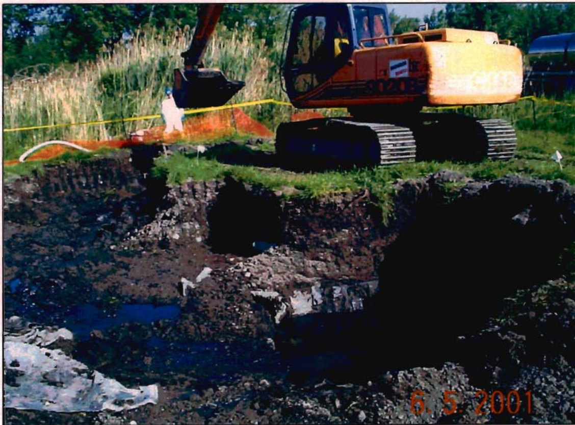
Groundwater seepage into excavation.
