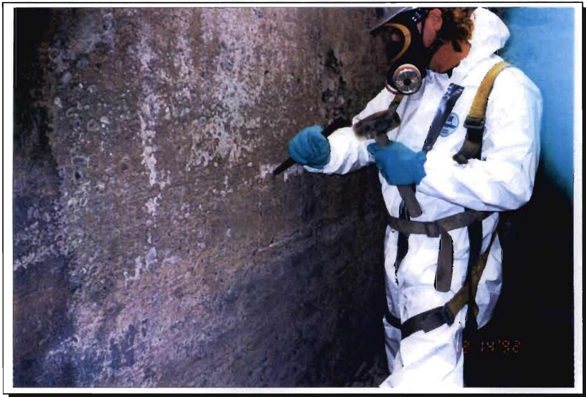
Photograph 11. Concrete chip sample.
