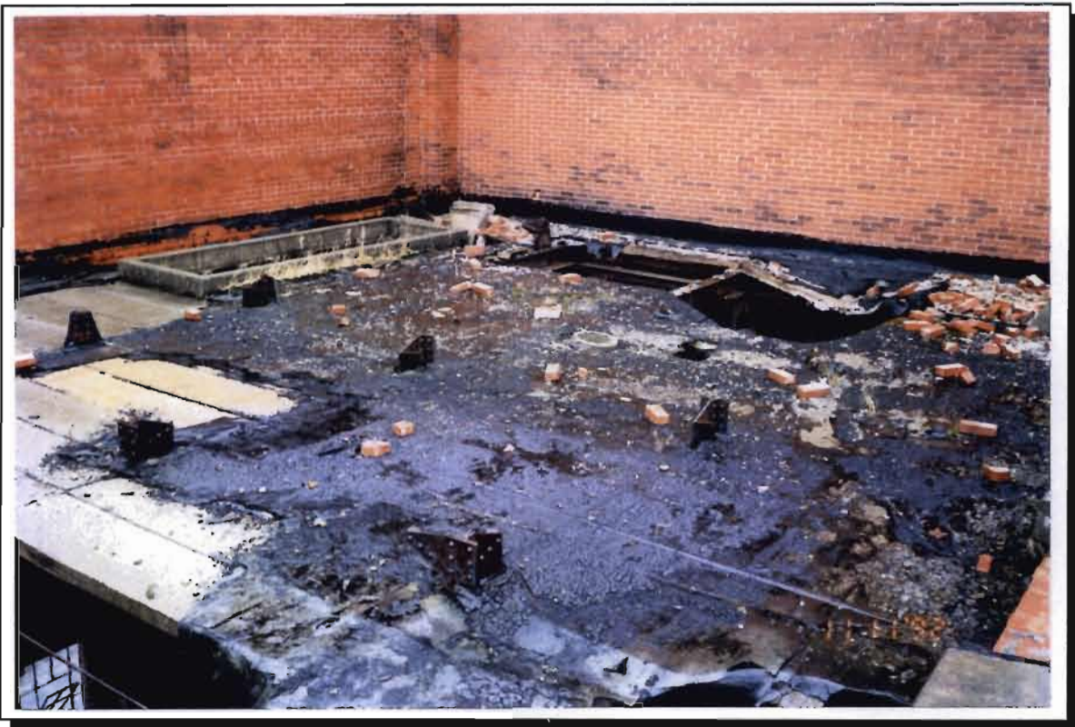
Photograph 2. Powerhouse roof on west side of building showing; (i) poor condition of roof; (ii) bricks from parapets; and (iii) non-friable asbestos material on some roof panels.
