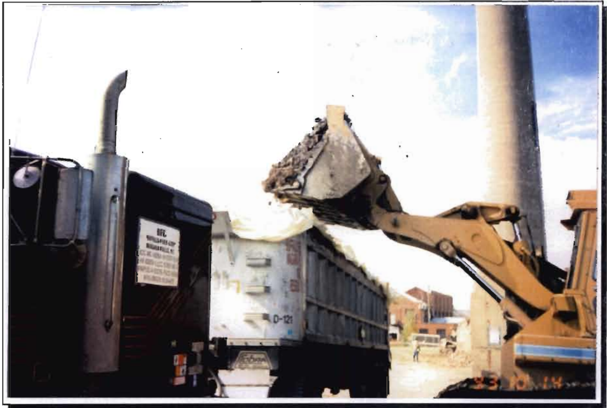
Photograph 9. Loading debris containing friable ACM into plastic lined units for transport to S&S Landfill.
