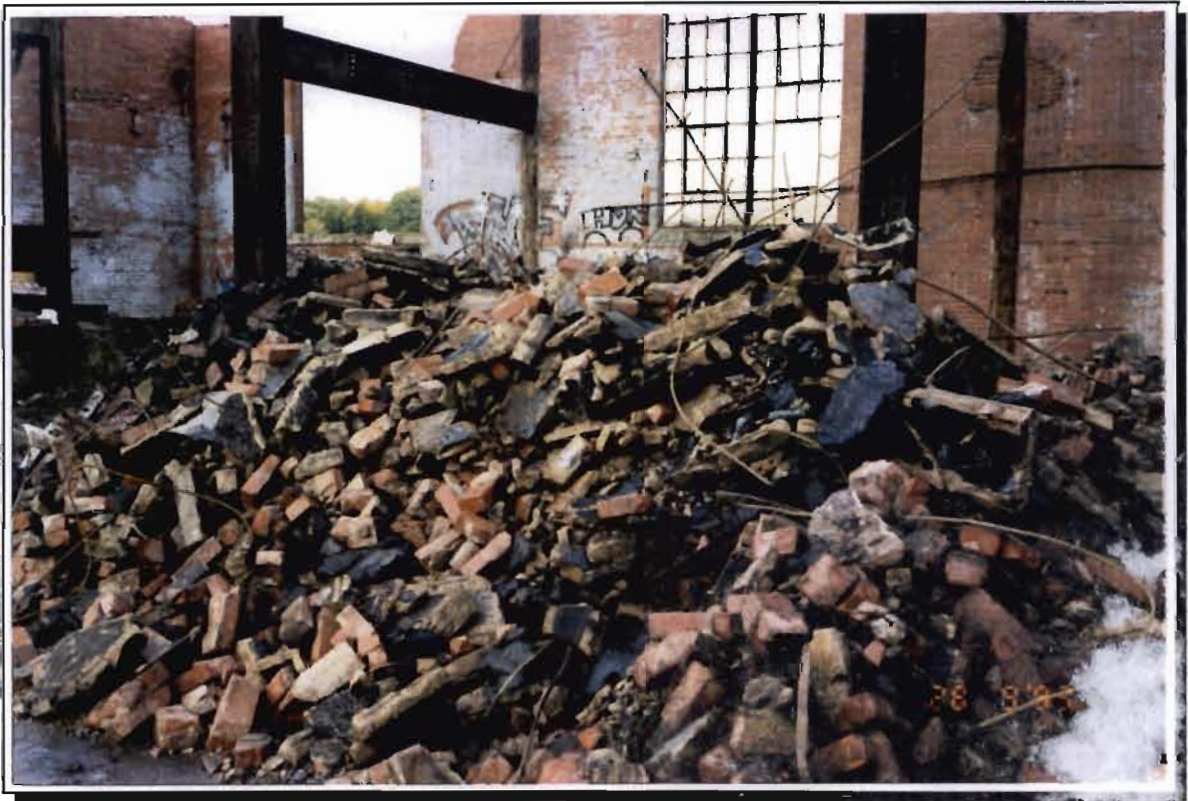
Photograph 8. Non-friable ACM mixed with clean debris at north end powerhouse.
