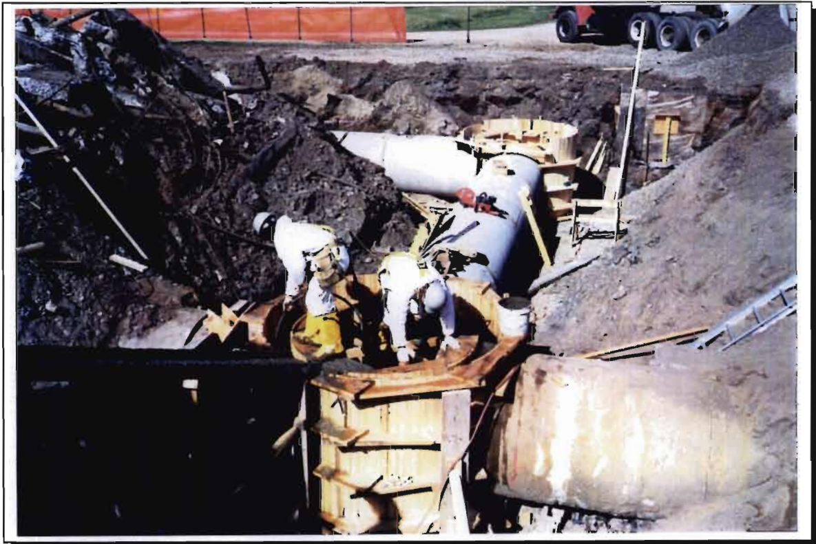
Photograph 5. Construction of by-pass sewer, showing construction of manhole MH-4 in foreground, on existing effluent line from separator, and manhole MH-3 in background.
