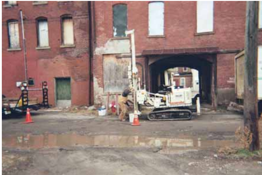
Date: 1/13/06 Subject: Direct-Push activities at the Band Box Cleaners Photographer: Jim Mays Site boring BB-BH-02
