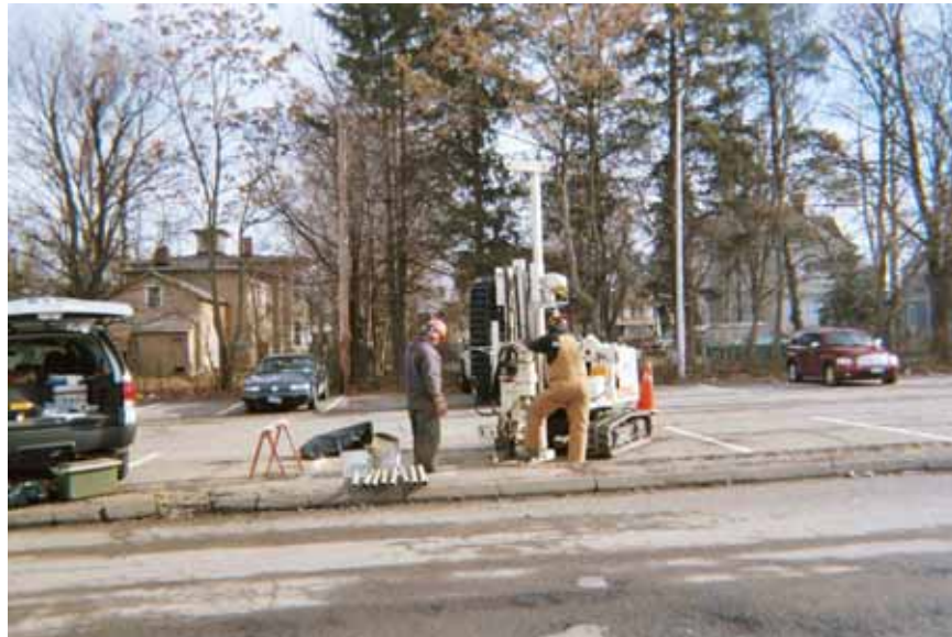
Date: 1/23/06 Subject: Direct-Push activities at the Former Liberty Street Dry Cleaners Site boring LS-BH-01 Photographer: Robert Meyers
