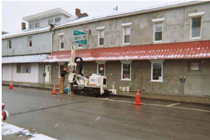
Date: 1/23/06 Subject: Direct-Push activities at the Former Liberty Street Dry Cleaners Site boring LS-BH-06 Photographer: Robert Meyers
