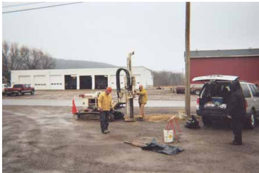
Date: 1/24/06 Subject: Direct-Push activities at the Canisteo Town Garage Site boring TG-BH-04 Photographer: Stephanie Reynolds Smith
