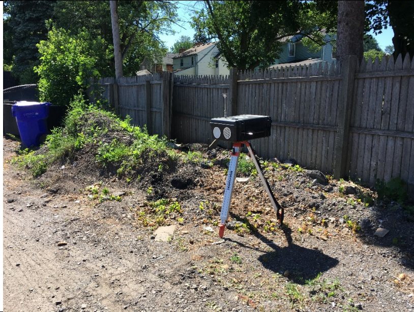
Title: Former Erwin Dry Cleaners Location: 1445 West Ridge Road, Greece, NY Date: June 14, 2018 Description: Typical Air Monitoring set-up (CAMP) in upwind and downwind locations to excavation area.
