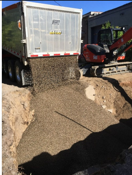
Title: Former Erwin Dry Cleaners Location: 1445 West Ridge Road, Greece, NY Date: June 15, 2018, 8:40 AM Description: Pea gravel was sed to backfill the bottom half of the excavated area.
