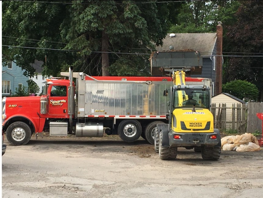
Title: Former Erwin Dry Cleaners Location: 1445 West Ridge Road, Greece, NY Date: June 21, 2018, 9:06 AM Description: Excavated soils being loaded into dump truck for off-site disposal.
