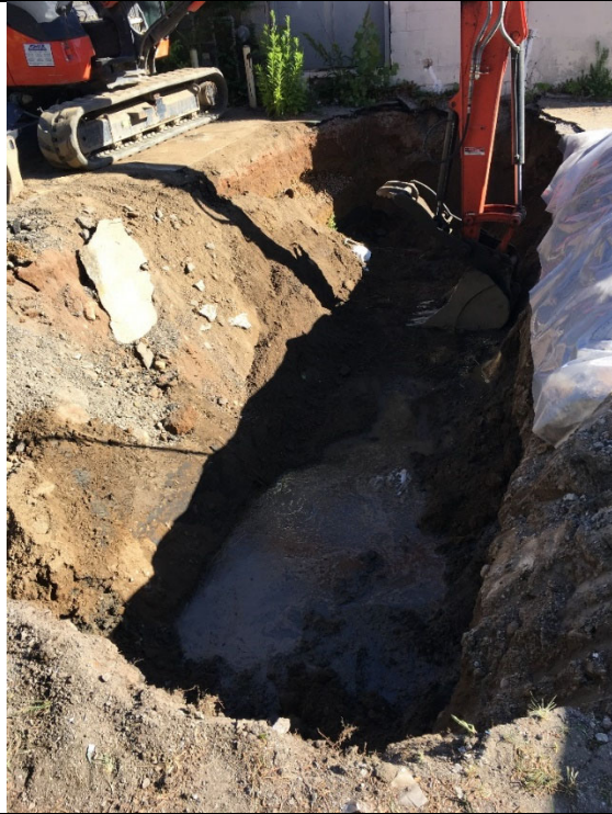
Title: Former Erwin Dry Cleaners Location: 1445 West Ridge Road, Greece, NY Date: June 15, 2018, 8:38 AM Description: Photo of excavated area after removal of UST and prior to backfilling.
