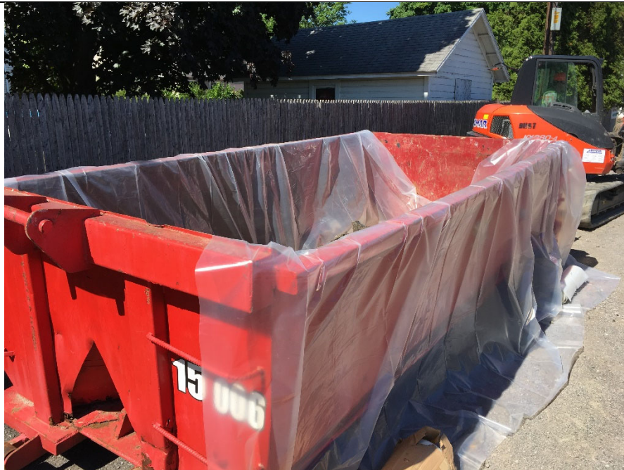
Title: Former Erwin Dry Cleaners Location: 1445 West Ridge Road, Greece, NY Date: June 14, 2018, 10:23 AM Description: Poly-lined roll-off container used to stage excavated soils for subsequent disposal.
