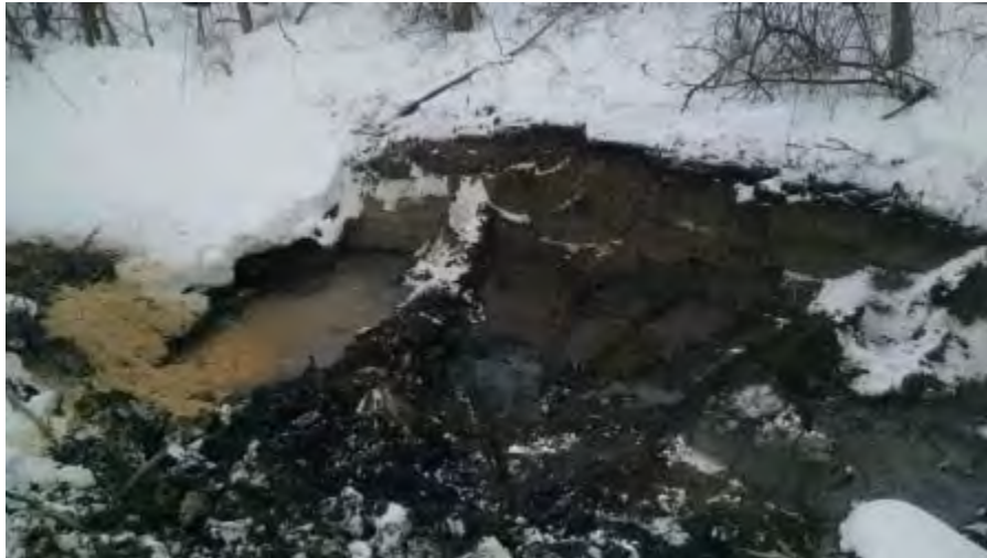
March 4, 2015 - View southwest, sawdust mixing with pooled water in southern end of excavation.
