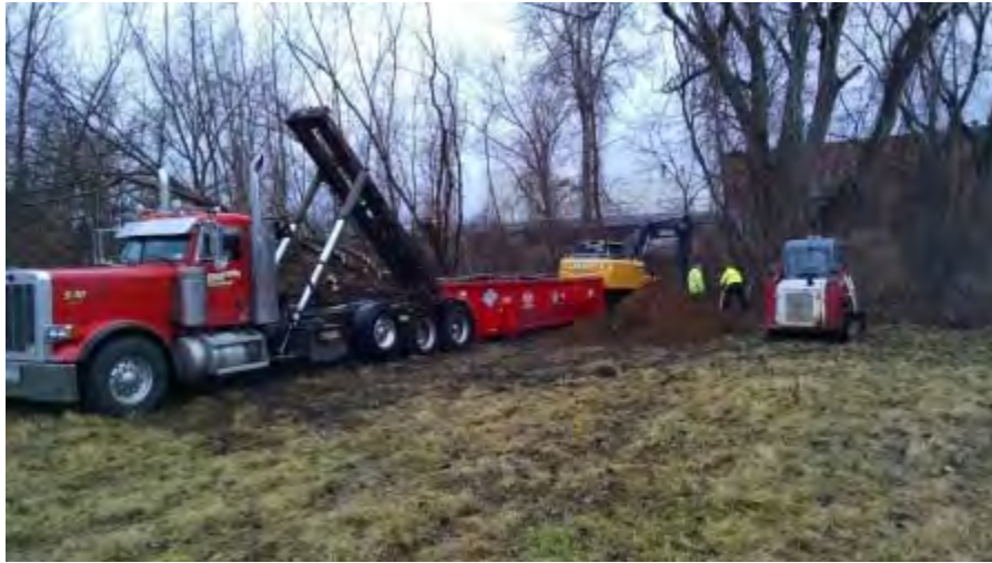
December 3, 2014 - View southwest, soil bin at excavation for immediate loading of discolored soil.
