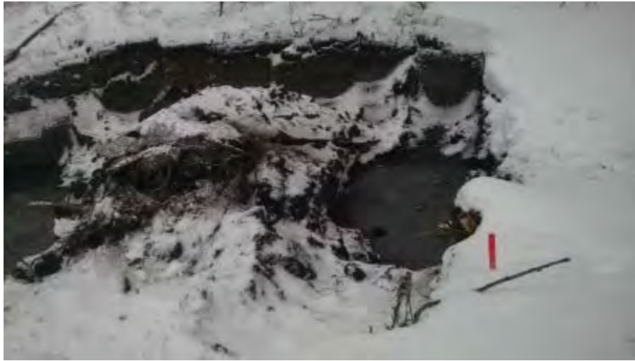
March 4, 2015 - View west, water pooling in the north side of excavation.
