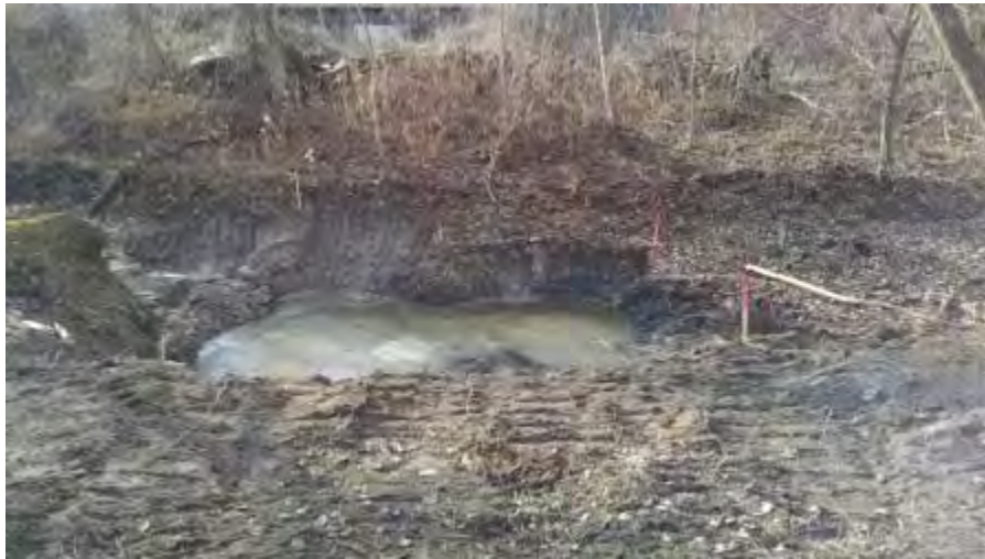
December 4, 2014 - View west, excavation at the end of the day backfilling with water.
