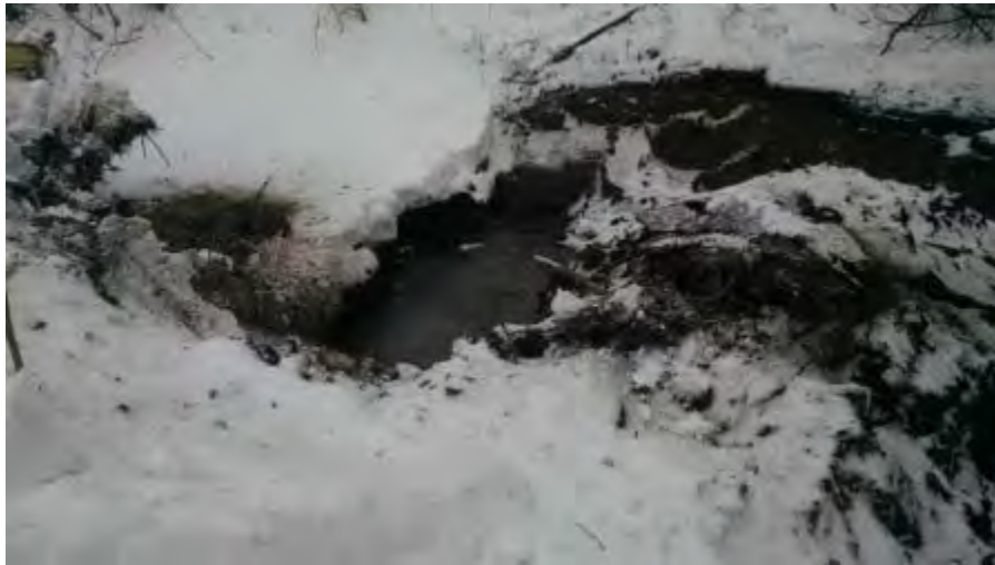
March 4, 2015 - View west, water pooling in the south side of excavation.
