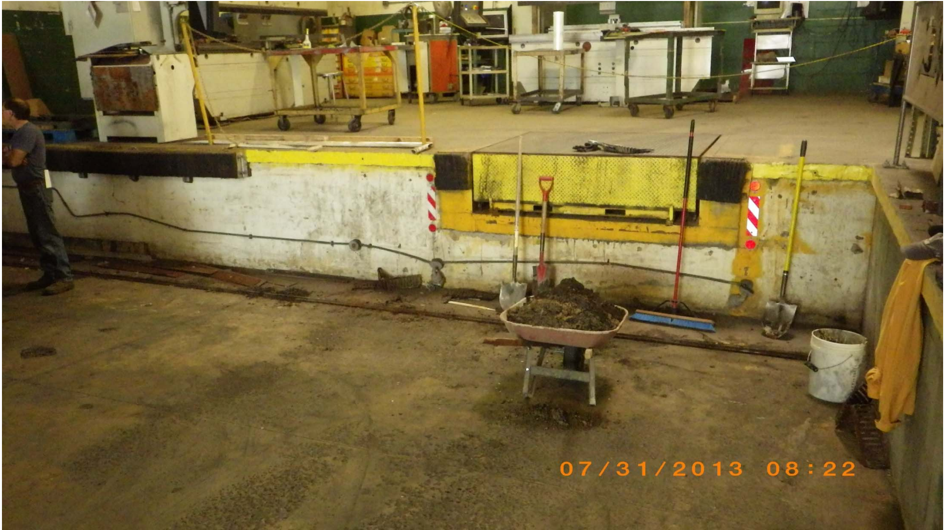
July 31, 2013 – Barthelmes Manufacturing: Closure of floor drains that discharge to the on-site stormwater basin located on west side of property. Image shows location of Trench Drain in loading dock area.
