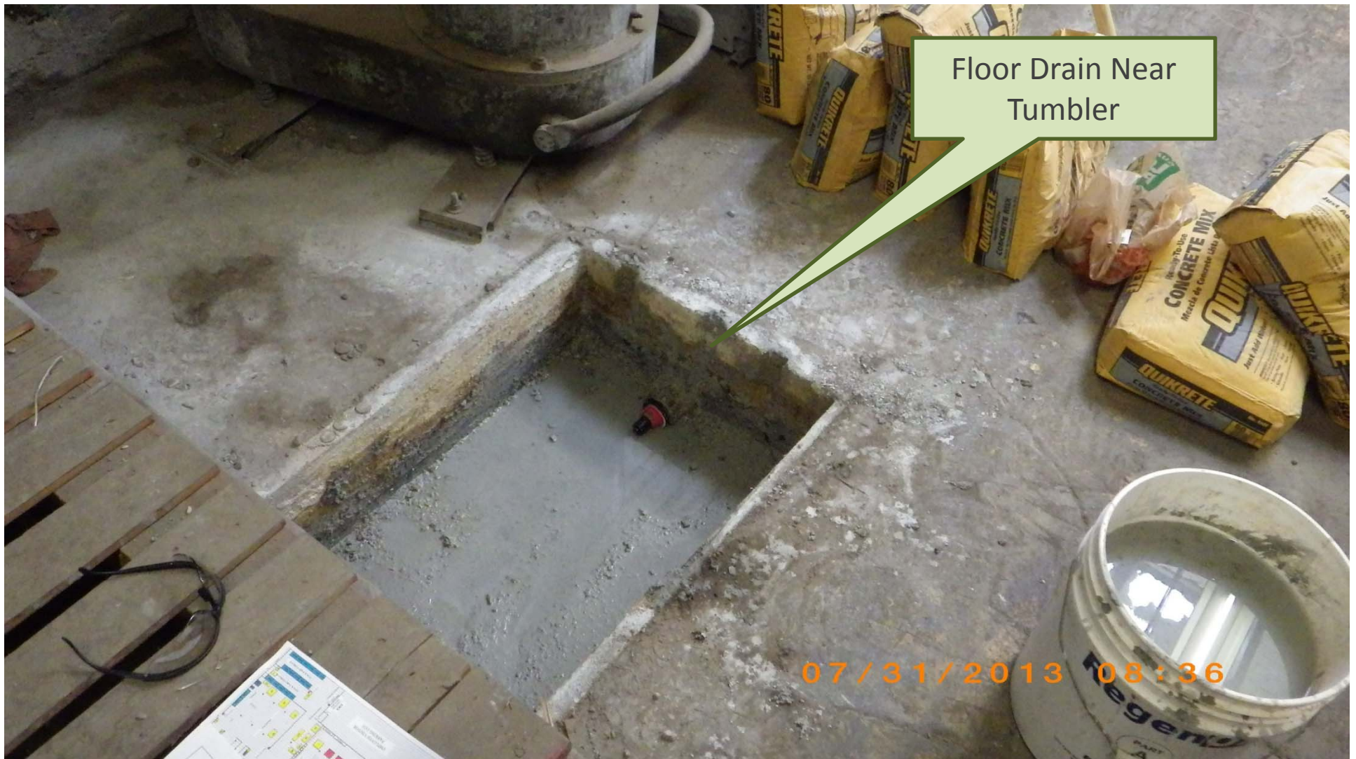
July 31, 2013 – Barthelmes Manufacturing: Closure of floor drains that discharge to the on-site stormwater basin located on west side of property. Plug placed in 2-inch drain pipe prior to cementing in-place.
