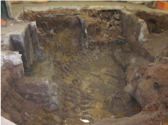
Photograph of southern portion of the former vapor degreaser left in place.
