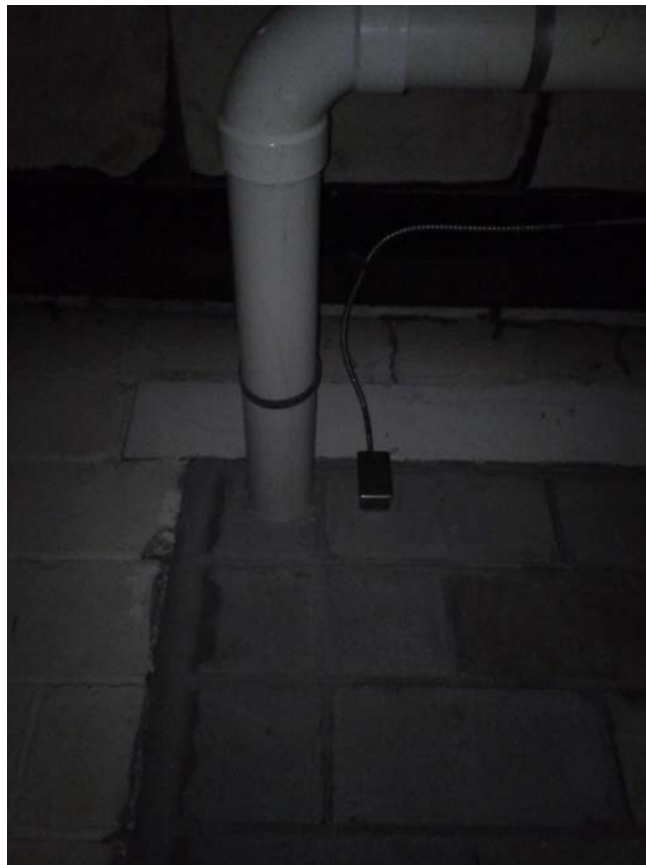
System 1 (North Room) Header and electrical
