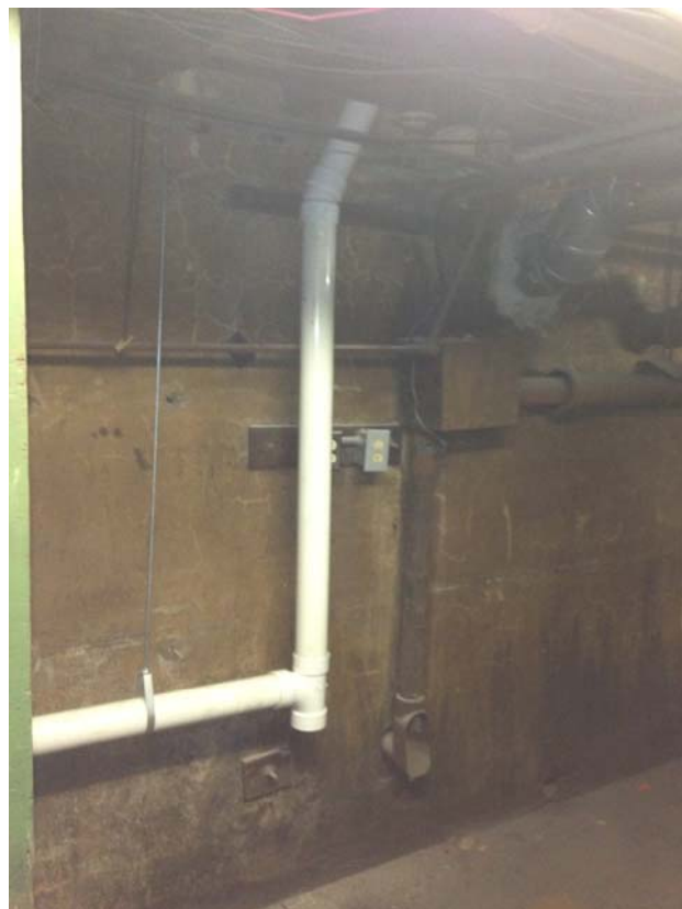
SP2 pre-connection to suction point and SP1 going through ceiling to furnace/electrical room.
