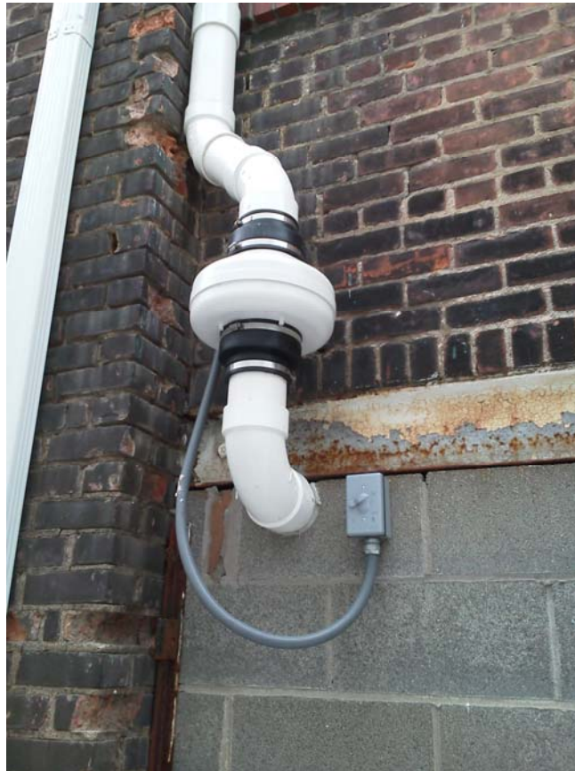
System 2 (Main System) RP 265 fan and switch
