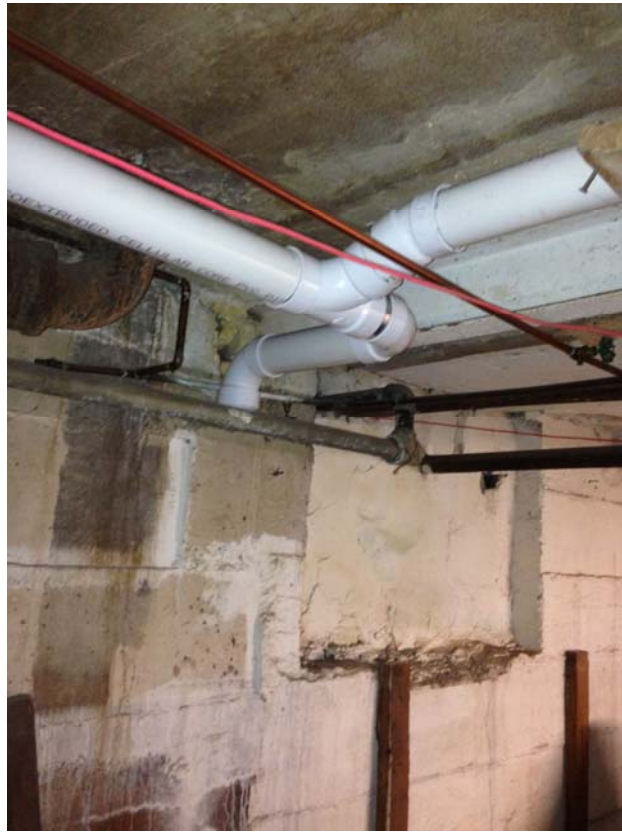
SP9 pre-vertical suction point connection and SP10 branching off to right.
