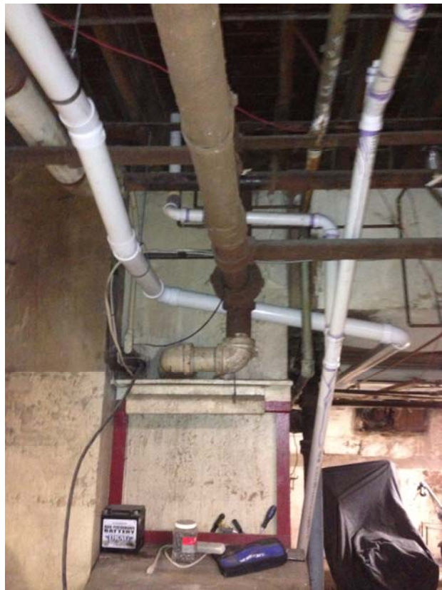
SP9 and SP10 branching off header.
