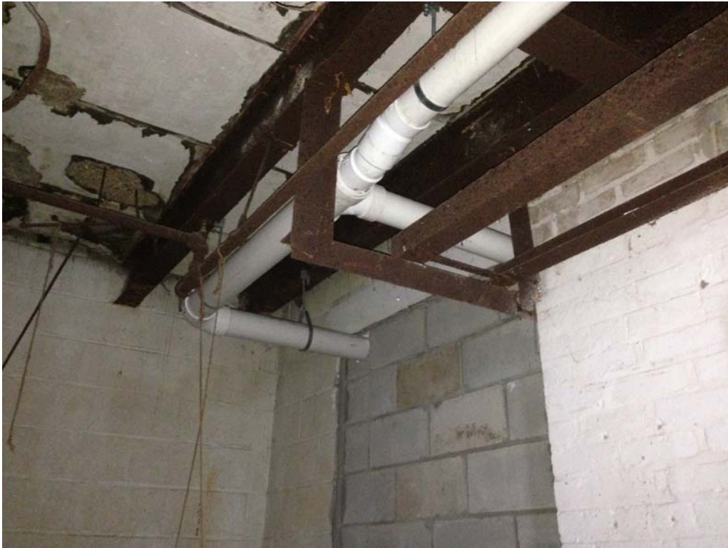
From left to right: System piping entering east side of Former RME facility, SP13 branching off and SP14 continuing.
