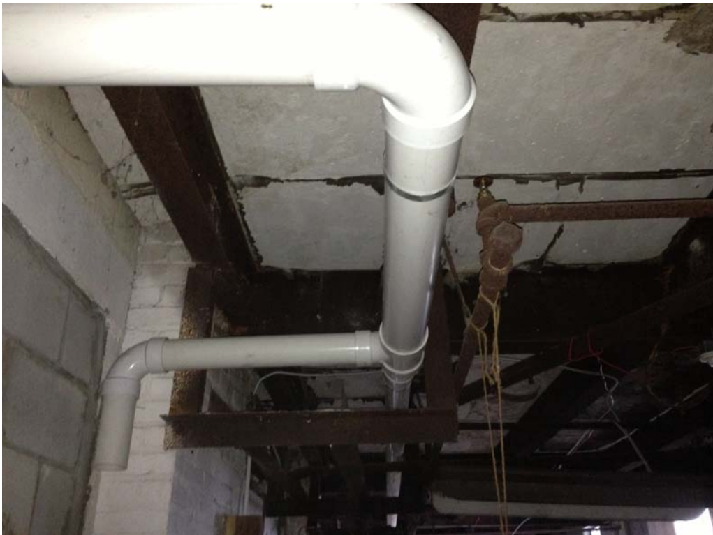
From top to bottom: SSD/SVE system entering east side of former RME facility, SP13 branching off and SP14 continuing.
