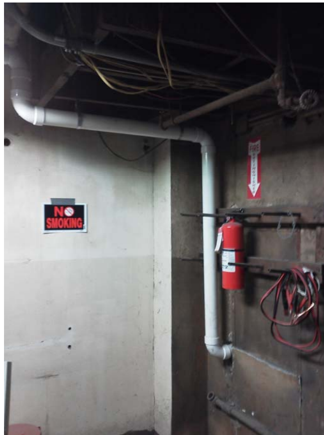
Piping to Suction Point 1 & 2
