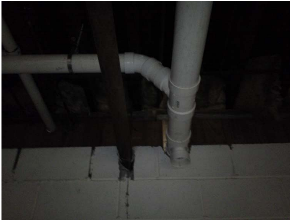
Main header entering main room. Also shown; SP6 and SP11 legs branching off.
