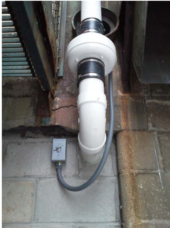
System 1 (North Room) RP 145 fan and switch
