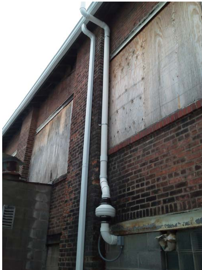
System 2 (Main System) RP 265 fan and exhaust stack
