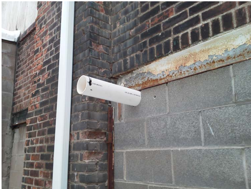
Main header entering east side of Former RME facility.
