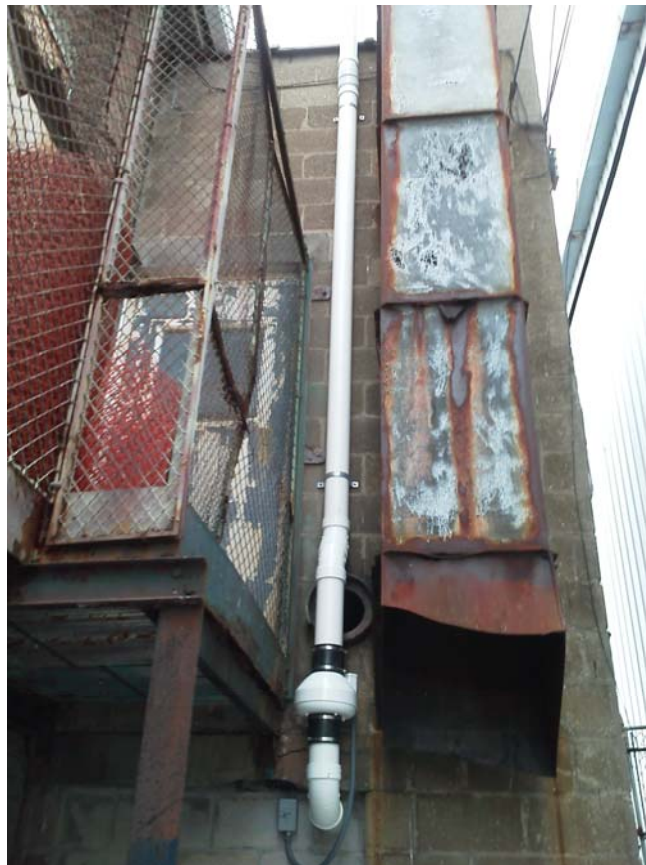
System 1 (North Room) RP 145 fan and effluent stack
