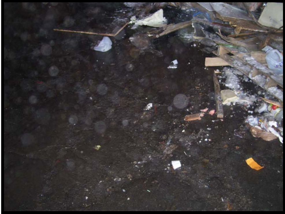
Location #50 – Large floor cracks
