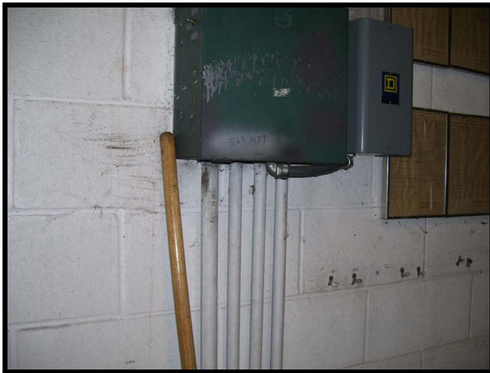
Location #4 – Conduit from floor in boiler room
