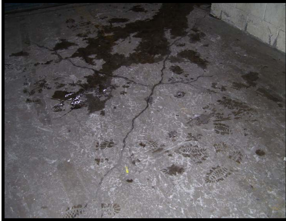
Location #1 – Crack in floor
