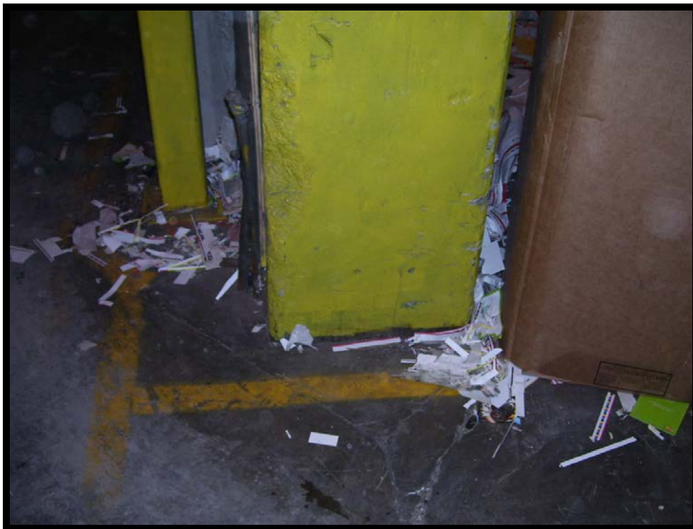
Locations #27 & 28 – Open conduit to floor near column/floor cracks near column
