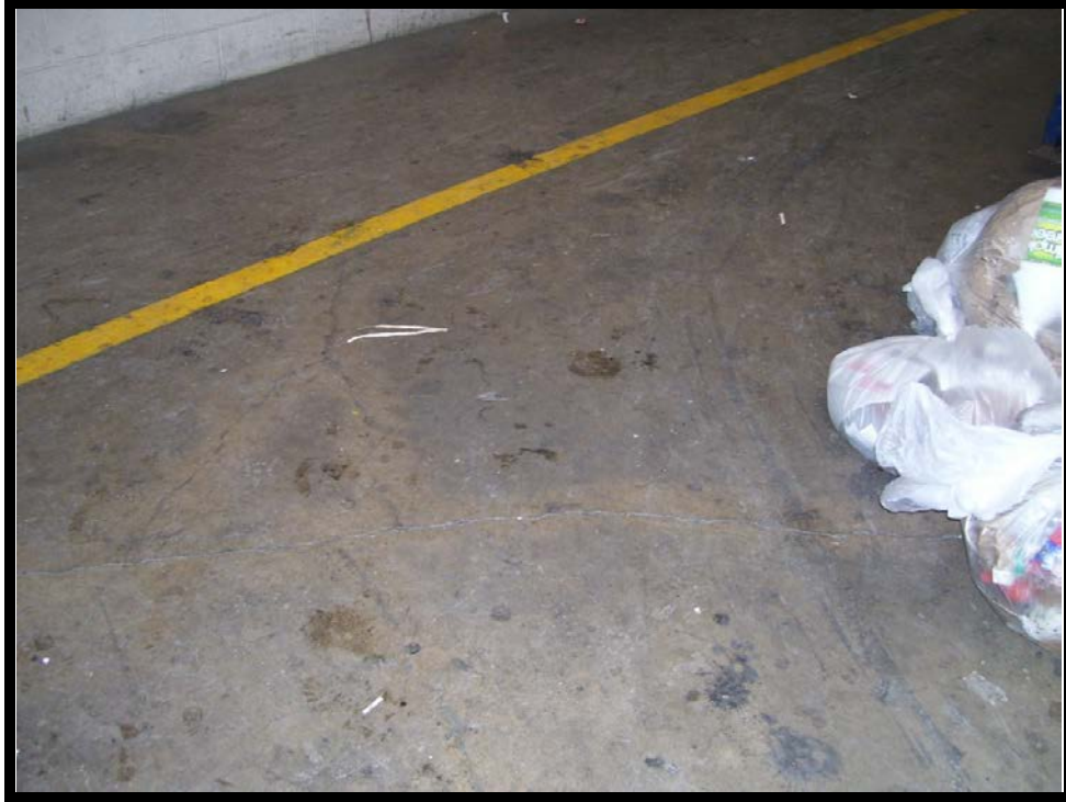
Location #11 – Floor cracking
