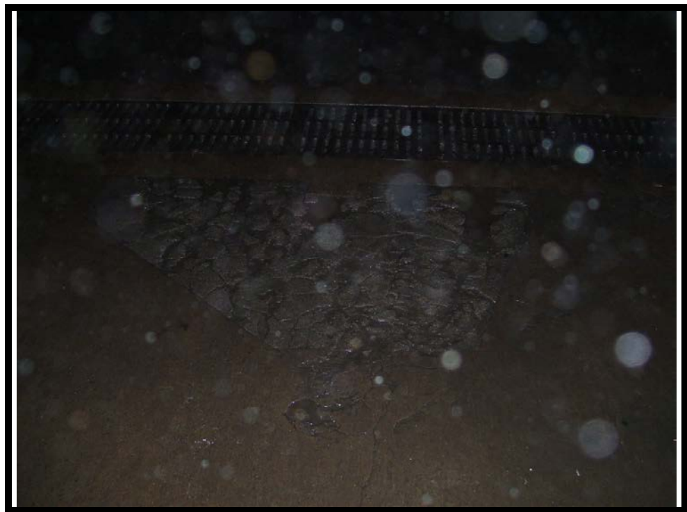
Location #58 – Floor cracks
