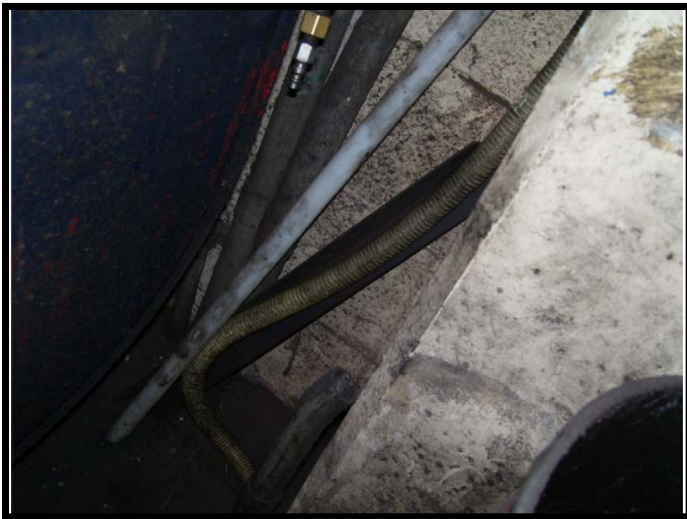
Location #22 – Open conduit to floor
