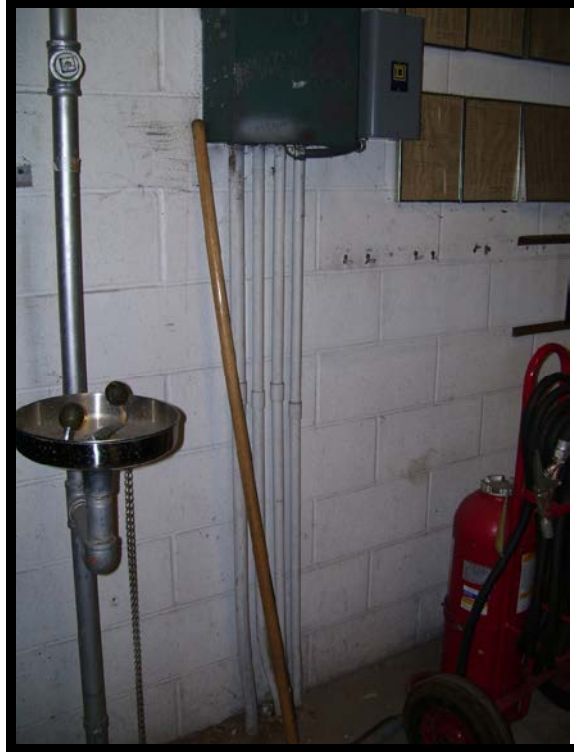
Location #4 – Conduit from floor in boiler room
