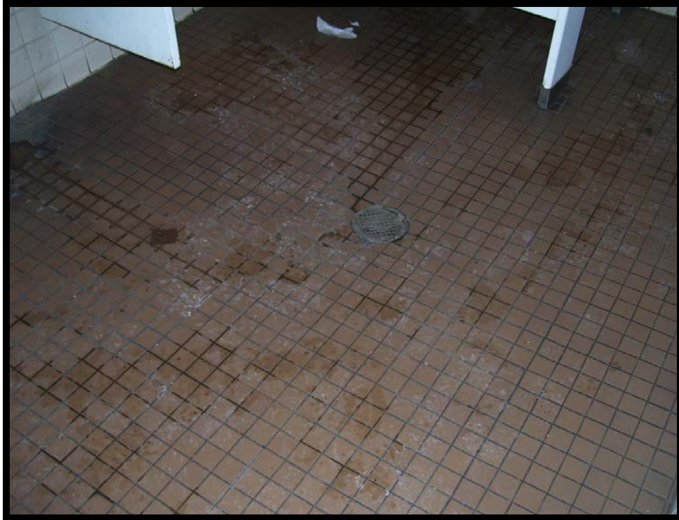
Location #92 – Floor drain men’s room (office area, base floor)
