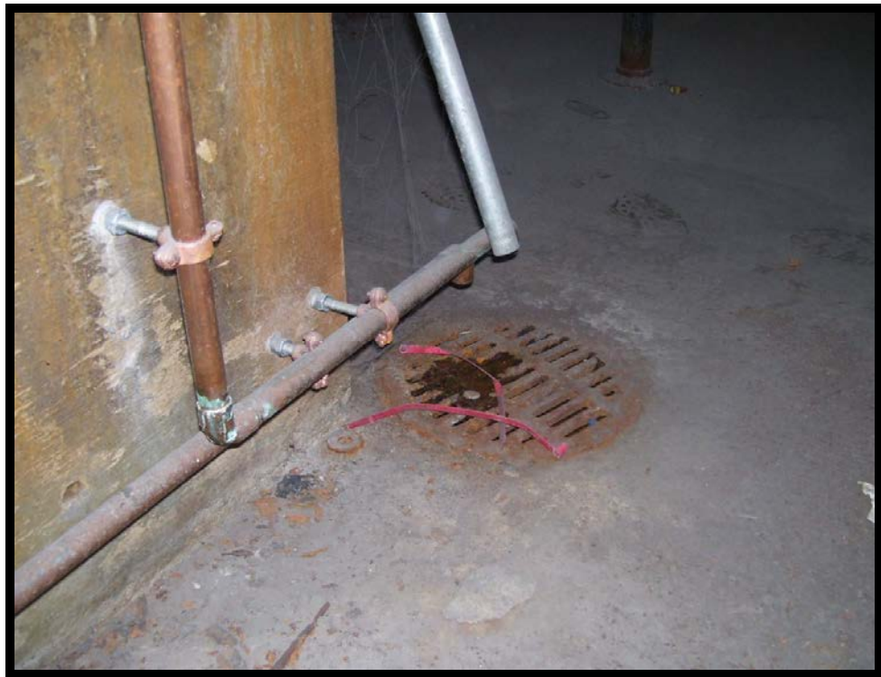
Location #47 – Floor drain in fire pump room
