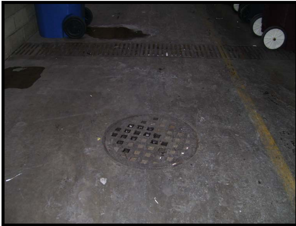
Location #32 – Manhole (oil interceptor)
