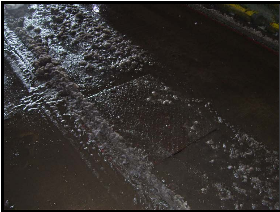
Location #36 – Scale pit
