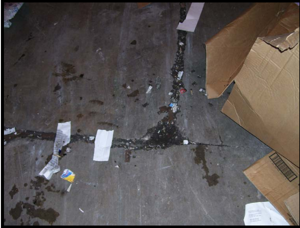
Location #26 – Large floor cracks
