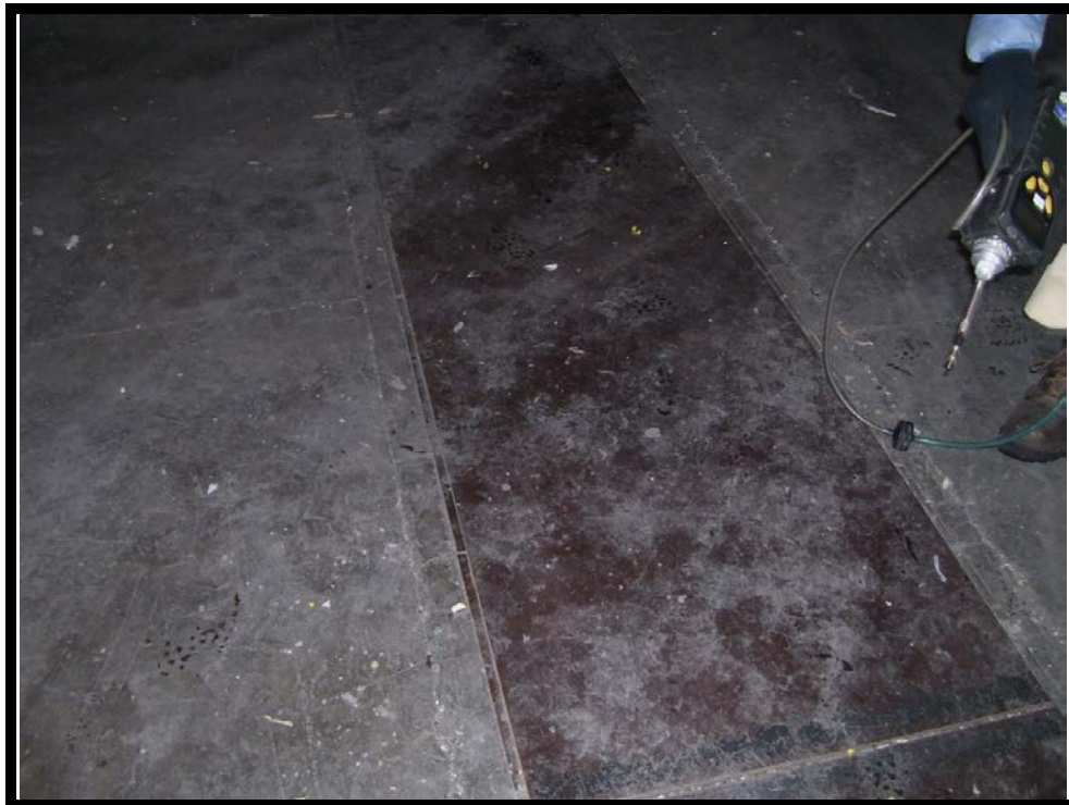
Location #86 – Hole in steel plate over vault
