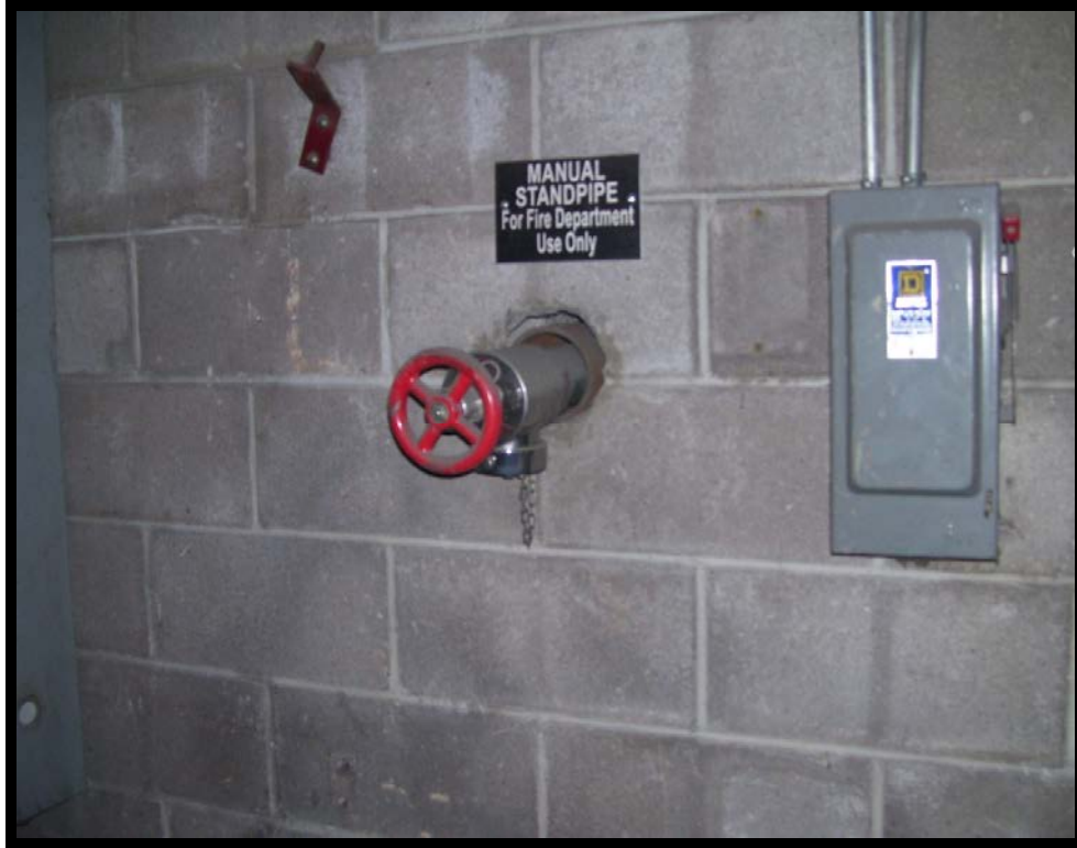
Location #117 – Electric room (manual standpipe)
