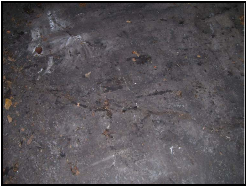
Location #65 – Floor cracks
