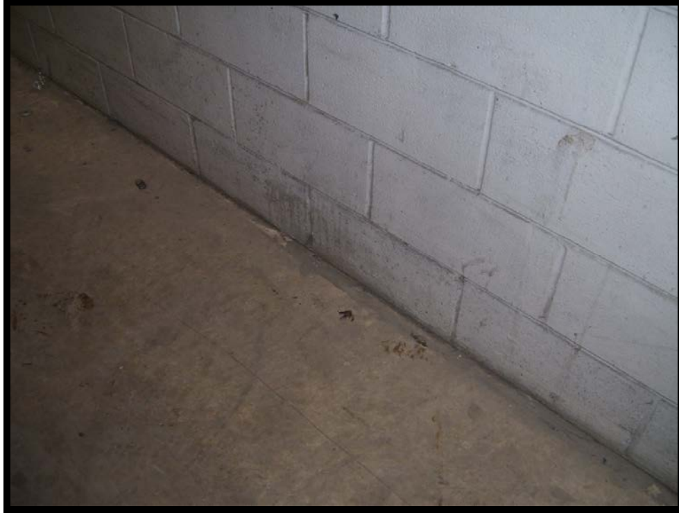
Location #15 – Wall/floor gap
