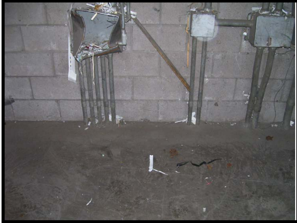
Location #98 – Floor/wall joint in RRF
