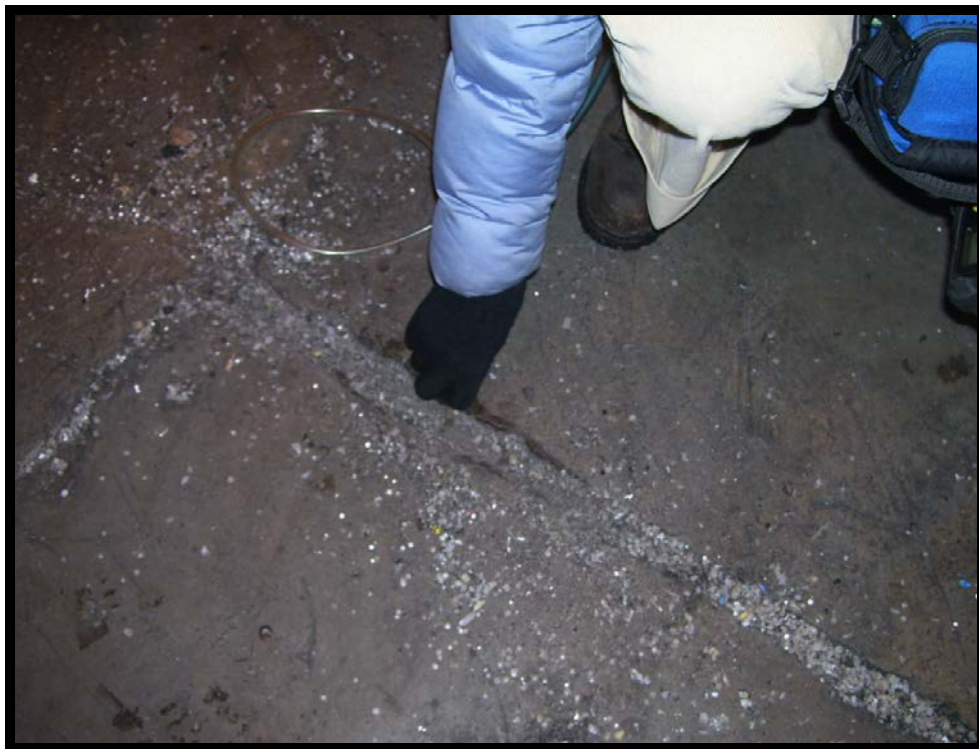
Location #88 – Floor crack
