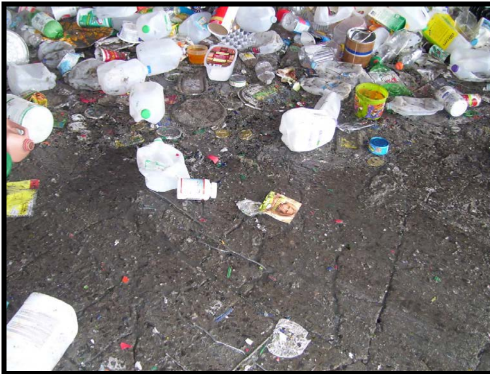
Location #80 – Broken concrete
