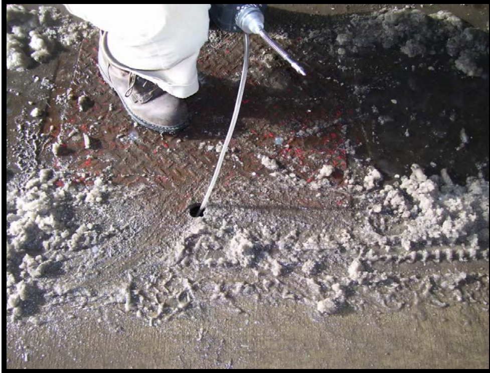
Location #35 – Scale pit
