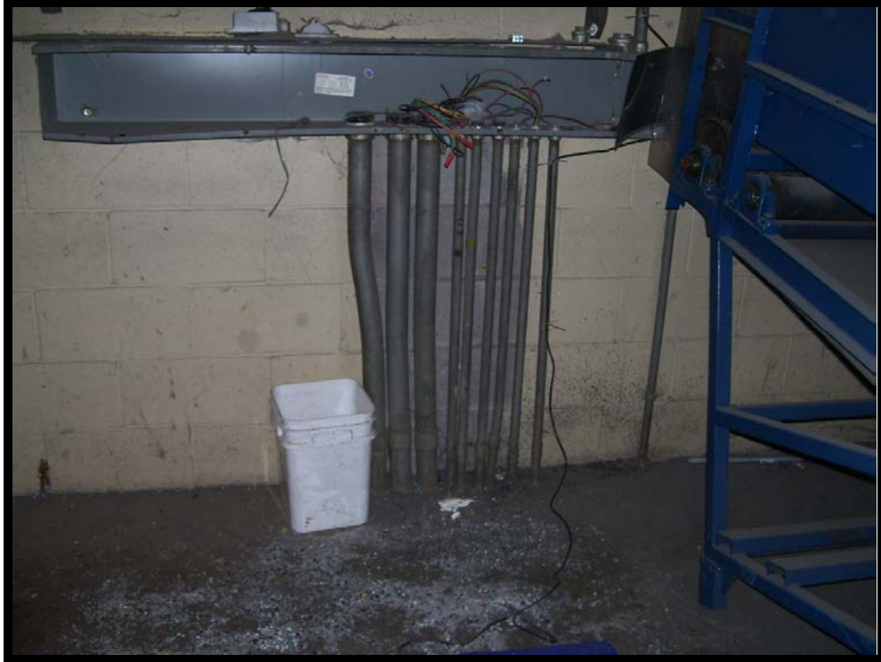
Location #90 – Open utility conduit
