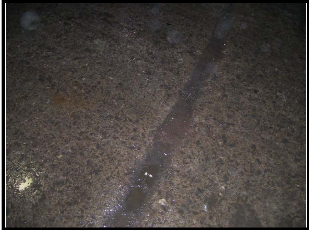
Location #57 – Floor joint
