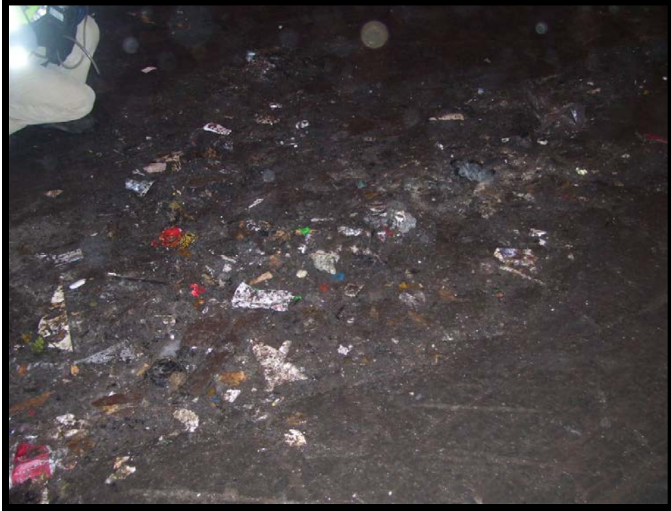
Location #63 – Floor cracks
