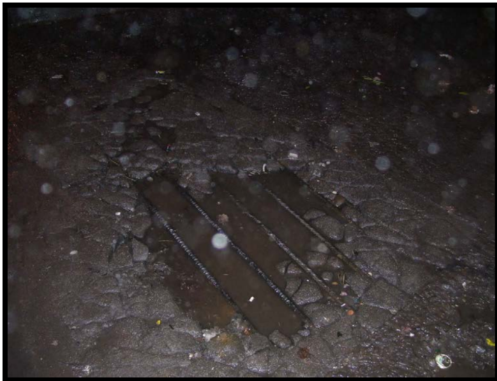
Location #60 – Broken floor
