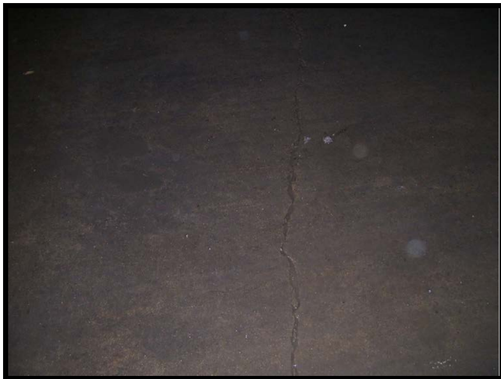
Location #43 – Large crack in floor
