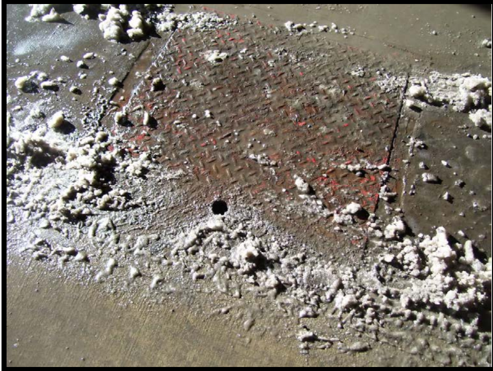
Location #38 – Scale pit
