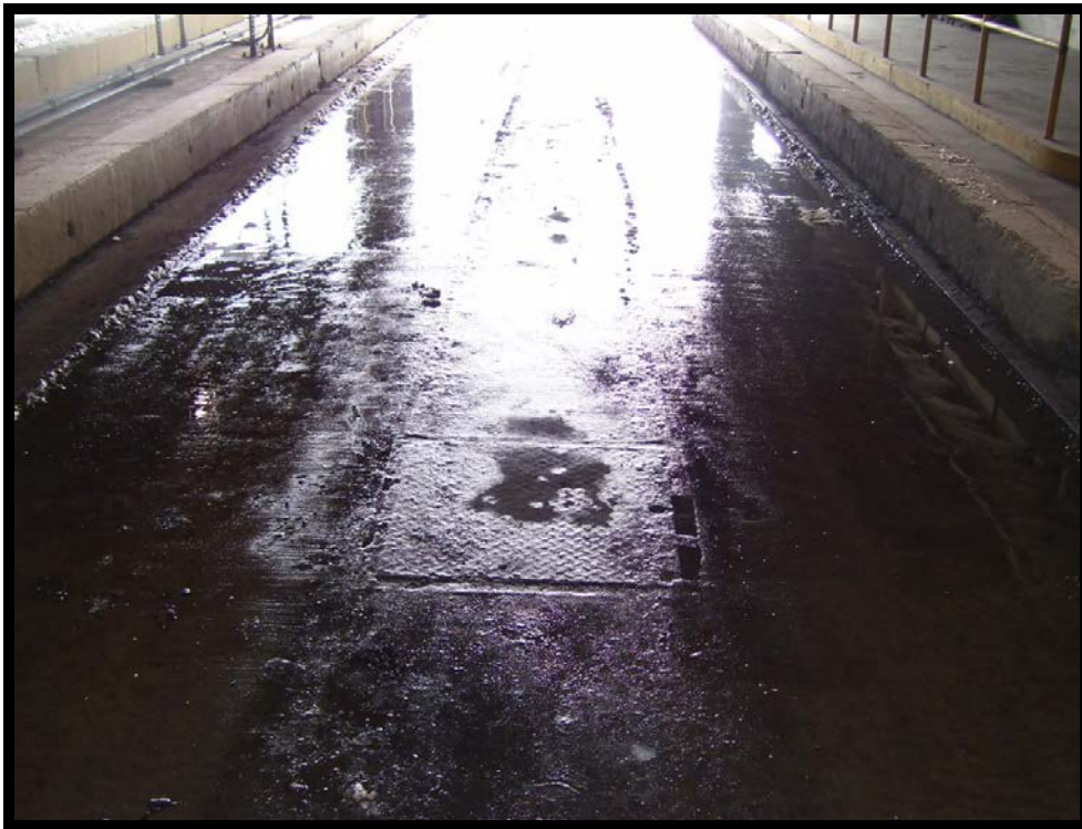
Location #34 – Scale pit
