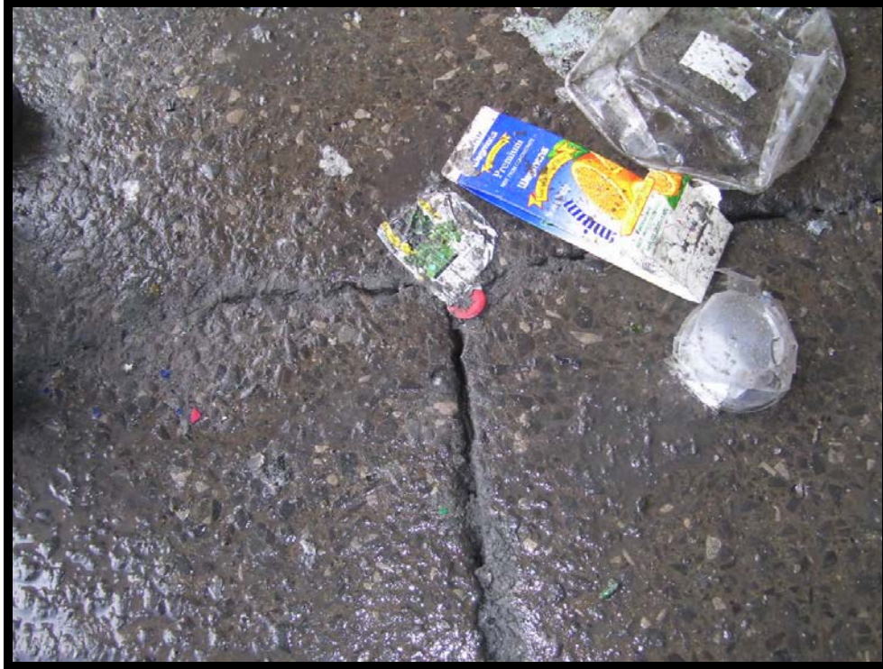
Location #79 – Floor cracks
