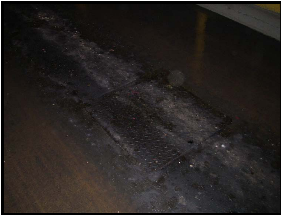
Location #39 – Scale pit
