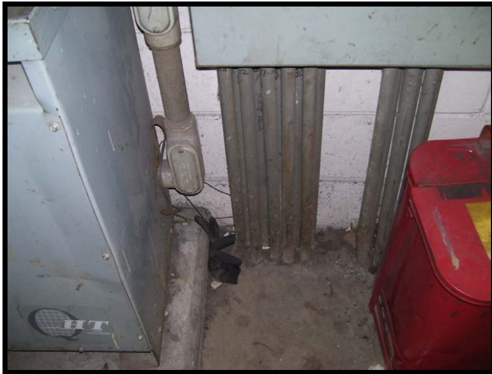
Location #16 – Conduit along wall
