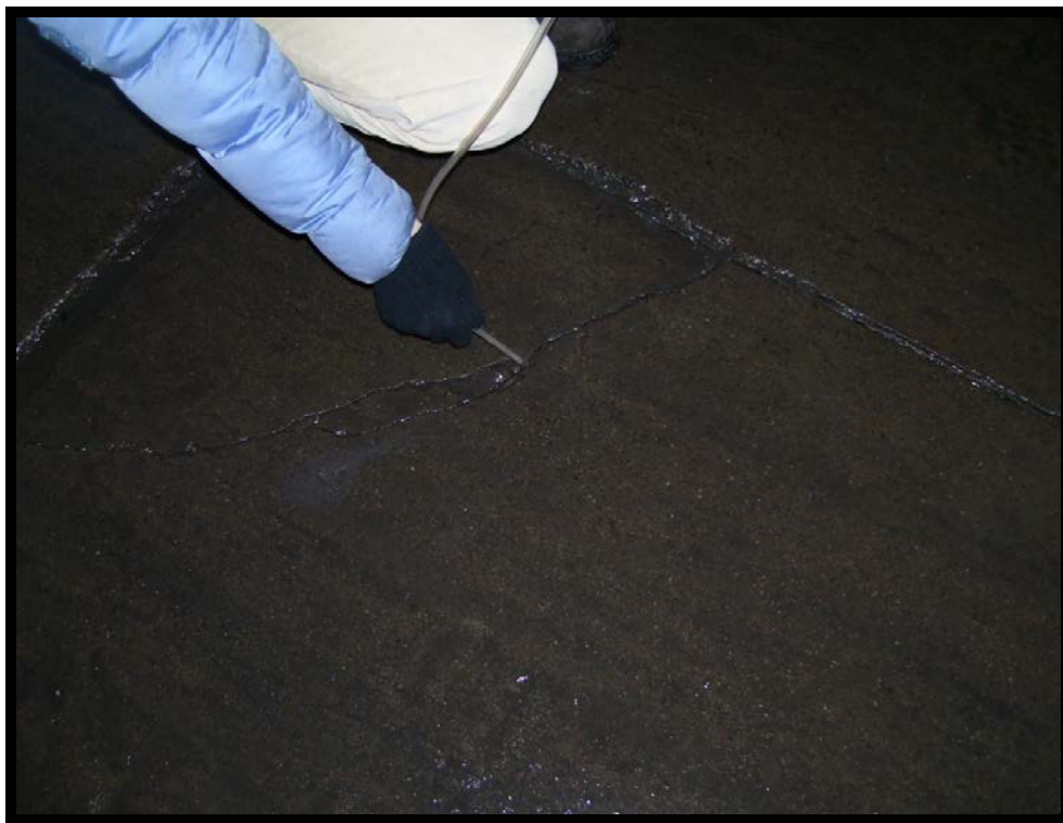
Location #41 – Large floor crack
