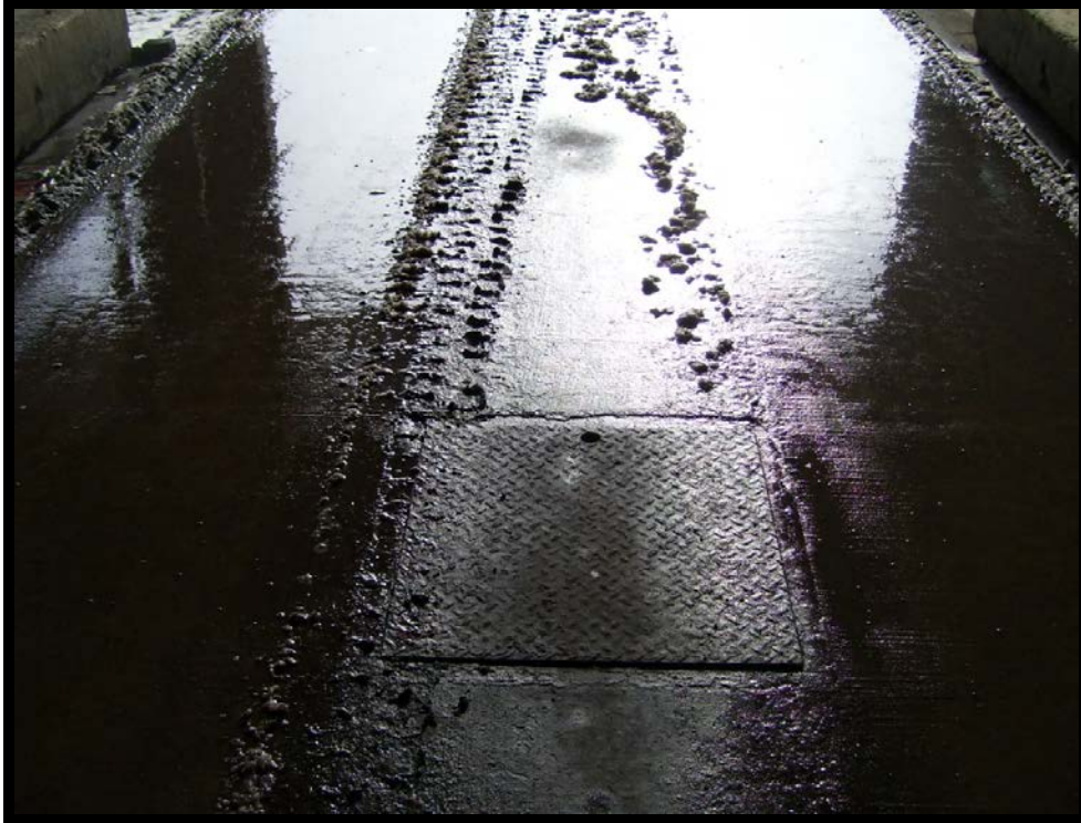
Location #33 – Scale pit
