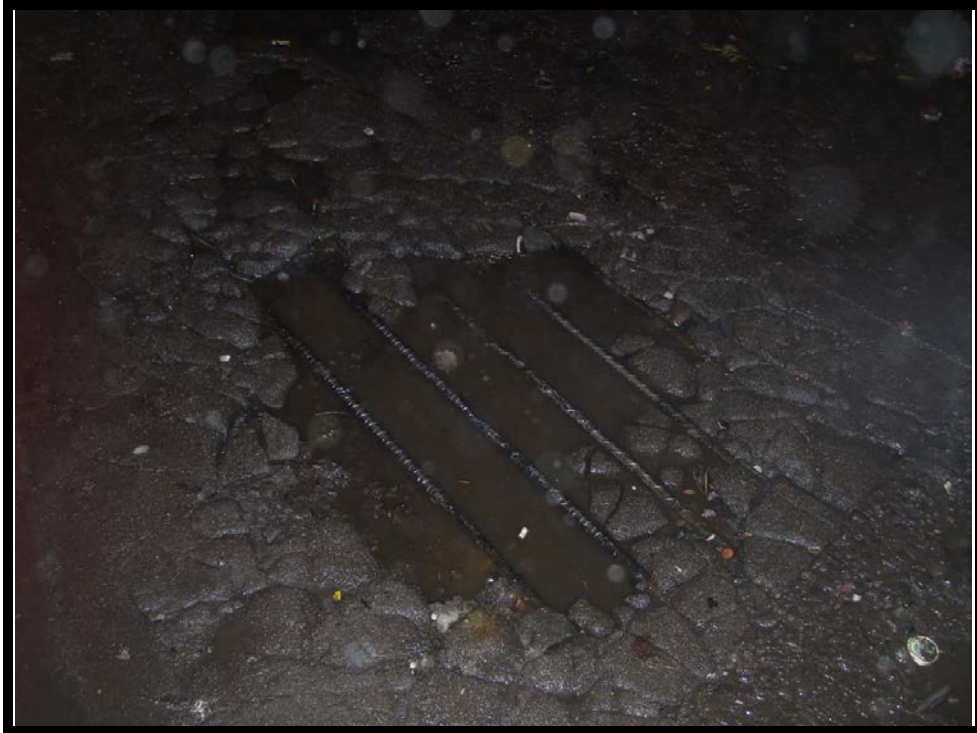
Location #59 – Broken floor
