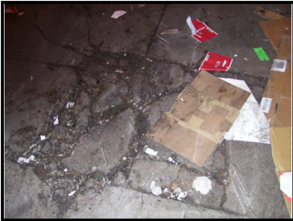
Location #25 – Large floor cracks
