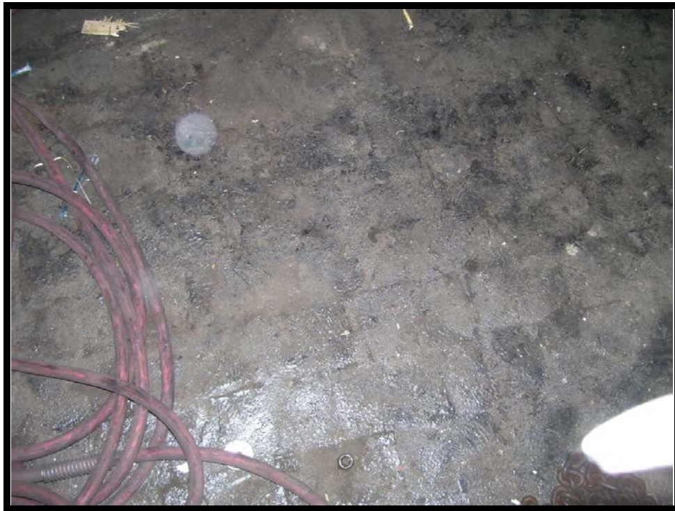
Wood block floor near flammable cabinet
