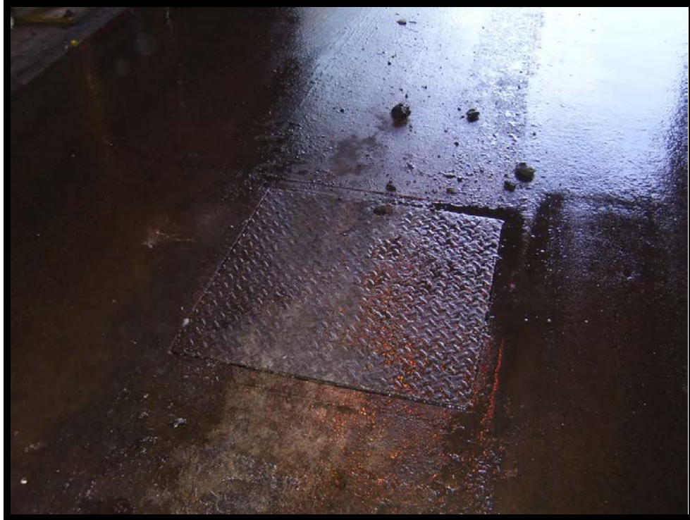
Location #40 – Scale pit
