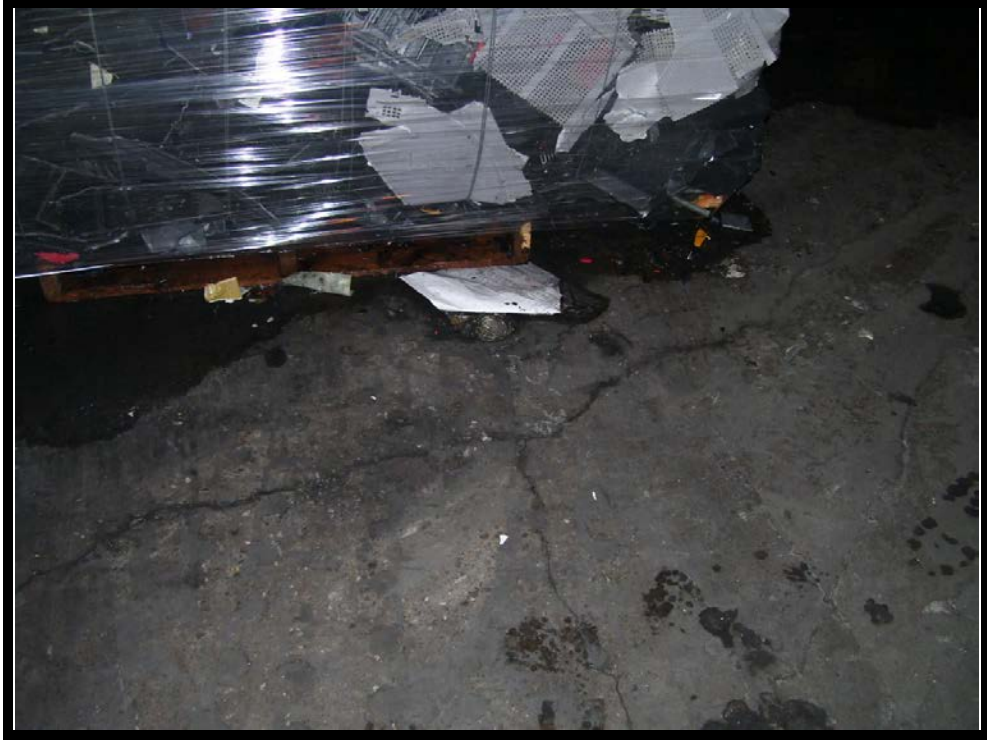
Location #70 – Floor crack
