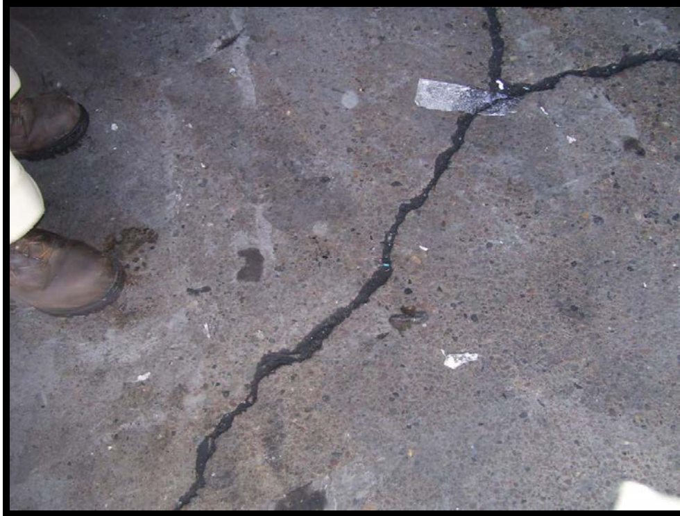
Location #81 – Floor crack
