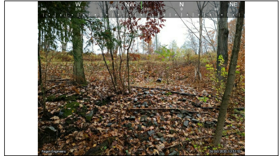
2.) Outfall of Sediment Trap 2. There have been no changes since last inspection.
