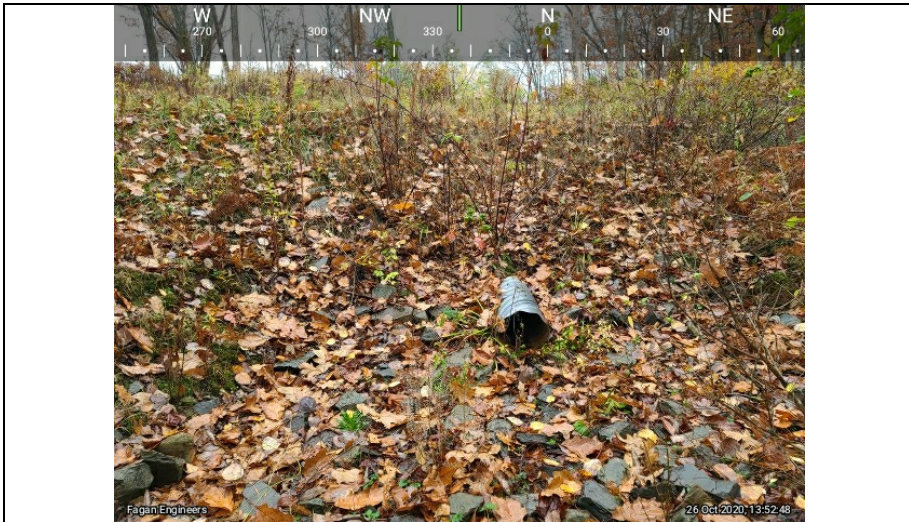
3.) A view of the Outfall Structure of Sediment Trap 2. There have been no changes since the last inspection.
