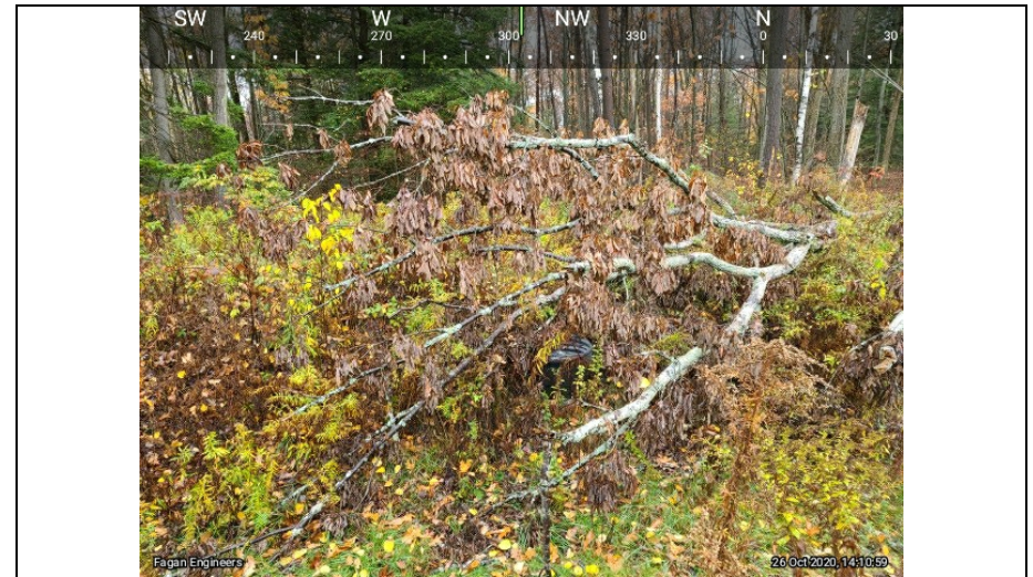
22.) A current view of outlet structure of sediment trap 1 note fallen tree.
