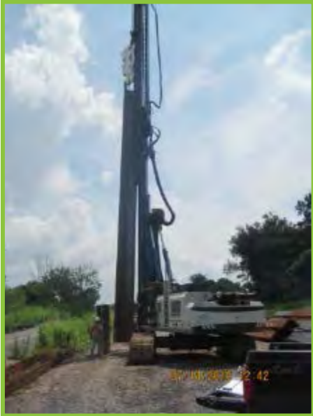
Figure 6: Installation of West Wall Portion of the Subsurface Sheet Pile Barrier Wall
