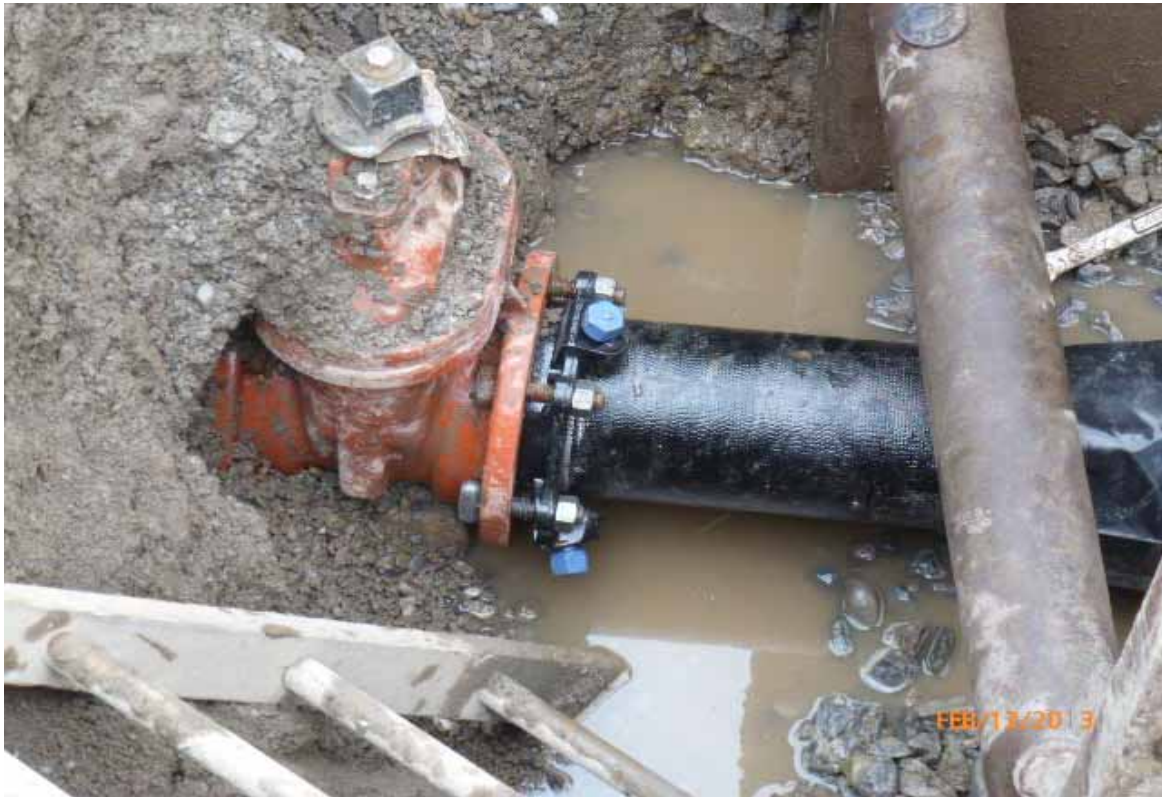
Photo #3: View of water around shutoff valve in water main installation trench southeast of monitoring well MW-11 (No Sheen Present)
