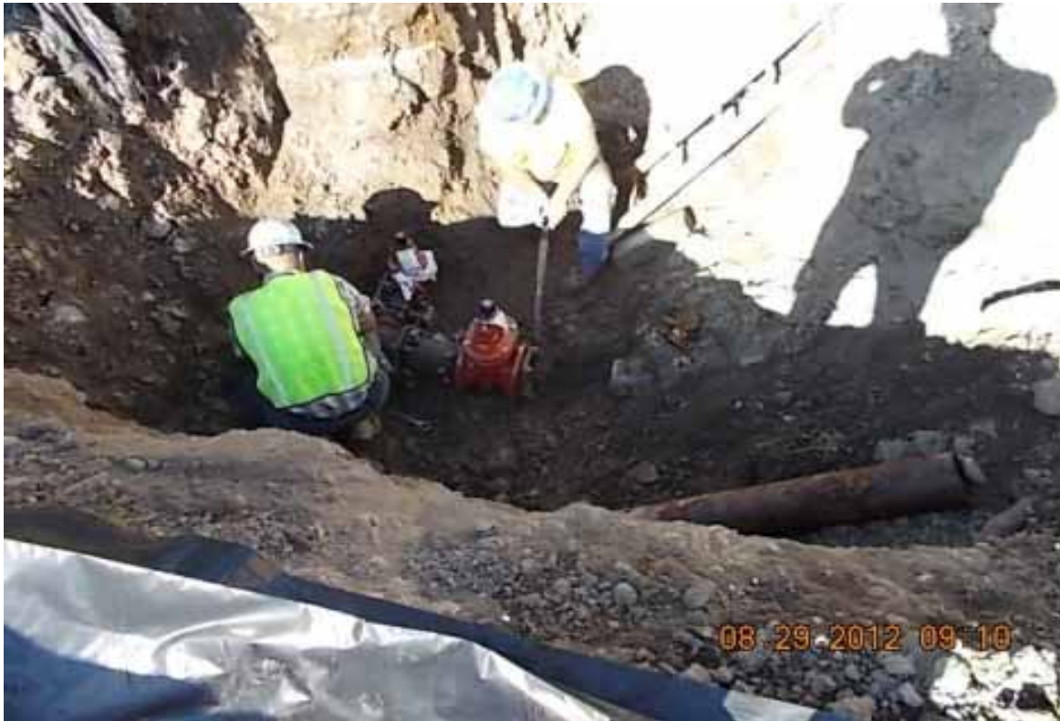
Photo #1: Installing water main shutoff valve and tee for the grout batch plant water supply line (Approximately 10 feet southeast of monitoring well MW-11)
