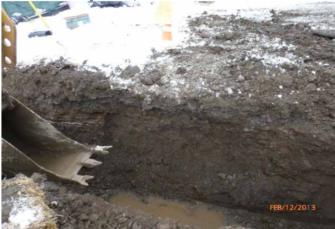
Photo #2: View of water main installation trench East of monitoring well MW-11 (cone with flag is on MW-11 cap)
