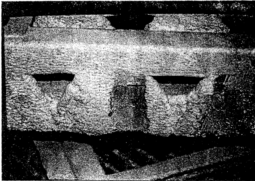
Figure 2. Fouling on trough distributor of an air stripper. Pour points can be severely plugged.
