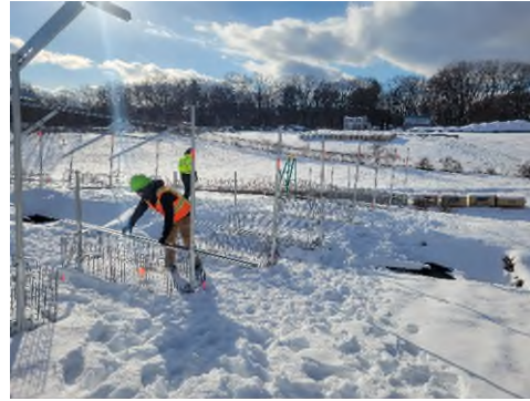
2. Baskets with racking braces removed from same area shown in photo #1.
