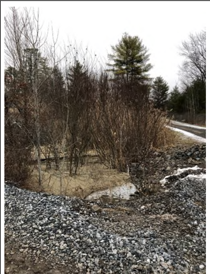
6. Sediment accumulation from initial erosion event in landfill perimeter swale.
