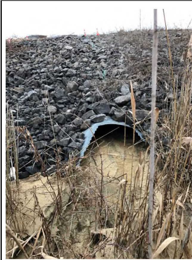
5. Sediment accumulation from initial erosion event in culvert that passes under landfill access road.
