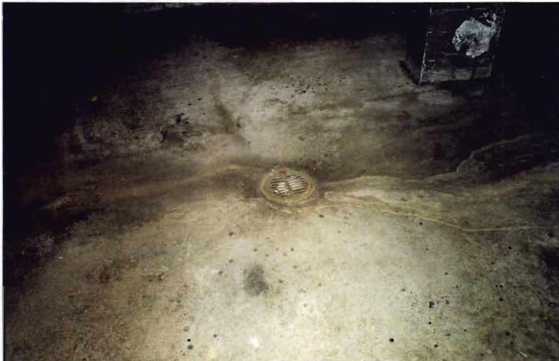
PHOTO 6 - A typical floor drain inside building 2820.
